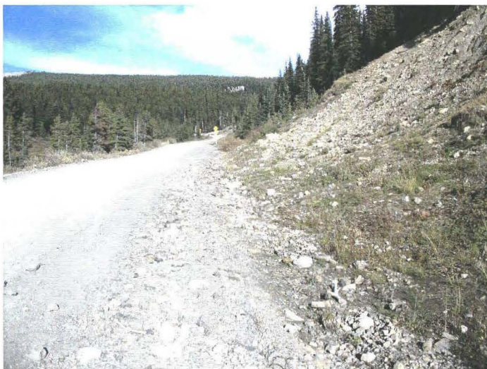
Photo 940-40 (bottom) – Closer view facing southbound along the toe of the slope. Note the accumulation of eroded material, including cobble-sized rocks, along the toe of the slope.
