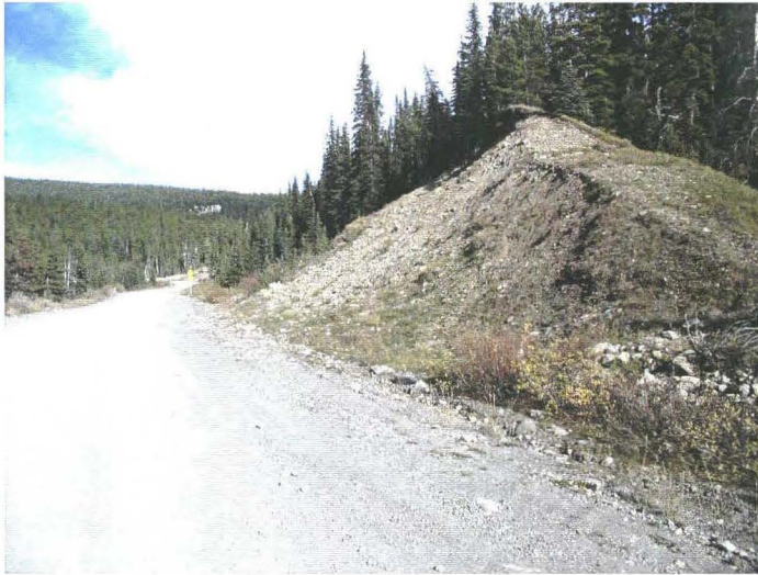
Photo 940-39 (top) – Facing southbound along the highway with the approximately 8 m high cut slope along the south side visible on the right. Note the lack of a ditch along the toe of the slope. The cut slope is marginally stable at 30 to 33° inclination, with eroded material from the exposed rocky soil rolling and sliding downslope to the road and accumulating along the toe of the slope.
