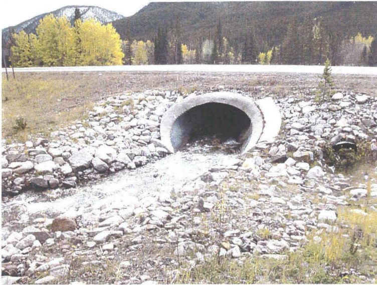
Photo 1 (top) – Facing downstream towards the culvert inlet at the Picklejar Creek crossing.
