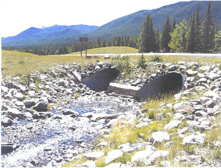
Photo 1 (top) – Culvert inlets at the Lantern Creek crossing. Both of these culverts have a series of vertical wood posts along the length of the culvert to prevent the culverts from being deformed by the weight of the overlying fill.
