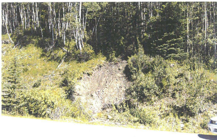
Photo 2 (bottom) – Shallow slump in the cut slope above the highway, approximately 10 m northwest of the culvert inlet. The debris from this slump was contained within the ditch.
