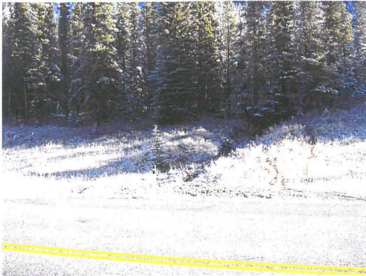
Photo 1 (top) – Fan of debris that has been deposited along the upslope (east) side of Highway 40 at an unnamed creek crossing approximately 1.8 km north of the Fortress Junction service station. The debris typically consisted of cobble sized rocks that appeared to have washed down along the creek channel during peak flows earlier in 2005.
