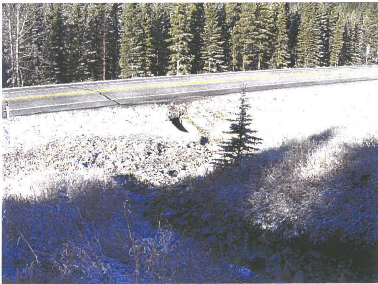
Photo 2 (bottom) – Facing downstream along the creek channel. The debris fan shown in Photo 1 is on the left side of this photo. Note how the culvert inlet is offset to the north (to the right, as seen in this photo) of the current position of the creek channel.
