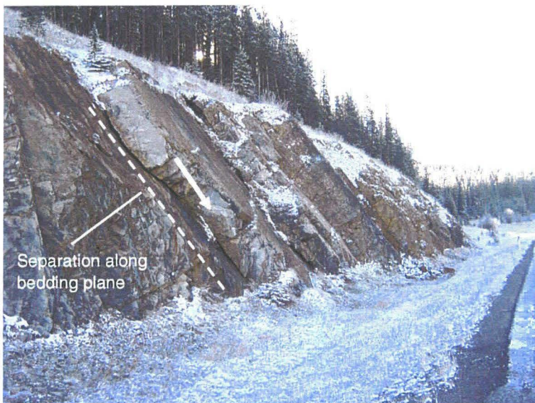
Photo 2 (middle) – Closer view of a segment of the rock cut slope showing separation along the exposed bedding planes. Water will flow into these gaps and freeze/thaw effects will cause the openings to grow larger during future years and also cause rockfalls due to weathering and breakup of the outer face of the cut slope. It is judged that the debris from such rockfalls will be contained within the ditch. It is possible that boulder-sized rocks will break off and slide down along the bedding planes, but they would be contained within the ditch.
