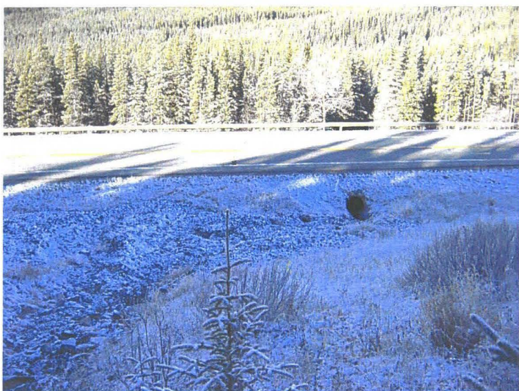
Photo 2 (middle) – Facing downstream along the creek channel. The debris fan shown in Photo 1 is on the left side of this photo. Note how the culvert inlet is offset to the north (to the right, as seen in this photo) of the current position of the creek channel.
