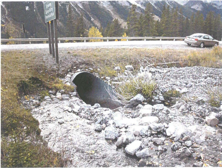
Photo 1 (top) – Facing west towards the culvert inlet at the Grizzly Creek crossing. The culvert itself was clear of debris at the time of the inspection, however a buildup of gravel to boulder-sized deposits along the channel immediately upstream of the inlet had raised the elevation of the base of the creek channel above the culvert base and deflected the creek flow a few metres to the south. This has resulted in erosion of the highway embankment sideslope immediately south of the culvert inlet. Note also the granular debris in the ditch and on the highway embankment sideslope to the north of the inlet (on the right hand side of the photo) – this debris appeared to have been deposited earlier in 2005.
