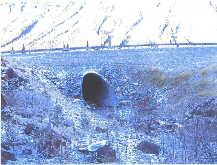
Photo 1 (top) – Facing the culvert inlet at the Ripple Rock Creek crossing. The diameter of the multiplate culvert is greater than 2 m and aside from a minor accumulation of gravel and cobbles near the inlet, it was completely clear of debris.
