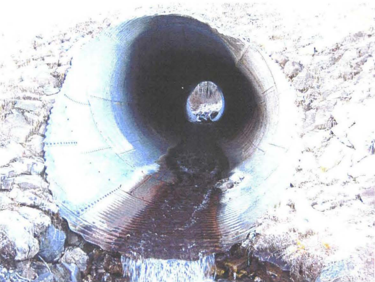
Photo 3 (bottom) – Facing upstream through the culvert at the Ripple Rock Creek crossing. There was a minor drop-off at the culvert outlet, however the channel below the culvert was well-armored and no signs of erosion that could undermine the culvert outlet were noted.
