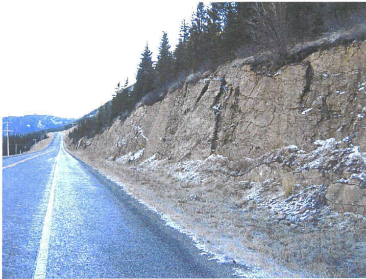
Photo 1 (top) – Facing north along a rock cut along the east side of Highway 40, between the Hood Creek and Ripple Rock Creek crossings. These cut slopes are approximately 4 to 5 m high and the near-vertical cut face exposes westerly-dipping, near-vertical bedding planes that are parallel to the highway. Minor volumes of rockfall debris have accumulated at the toe of the cut slope over time. At the time of the inspection there were no rocks on the road or signs of damage to the pavement from previous rockfalls.
