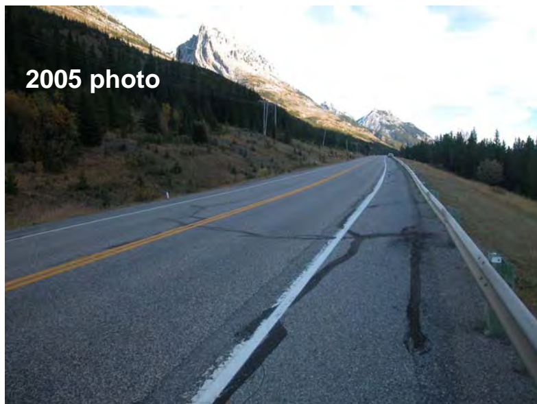
Photo 4 (bottom) – 2005 Fortress Junction Road Cracking Site The same area as shown in Photo 3, as it appeared during the 2005 inspection.
