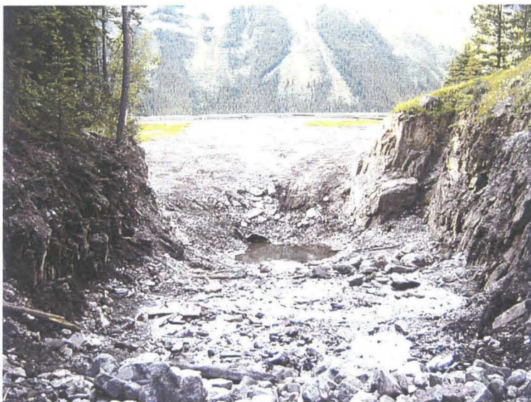
Photo 2 (bottom) – Facing downstream towards the culvert inlet. The culvert inlet was approximately 50% blocked with debris at the time of the July 2005 site inspection and it appeared that the culvert was fully blocked with debris further in. The low volume of creek flow at the time of the inspection was percolating through the debris in the culvert.
