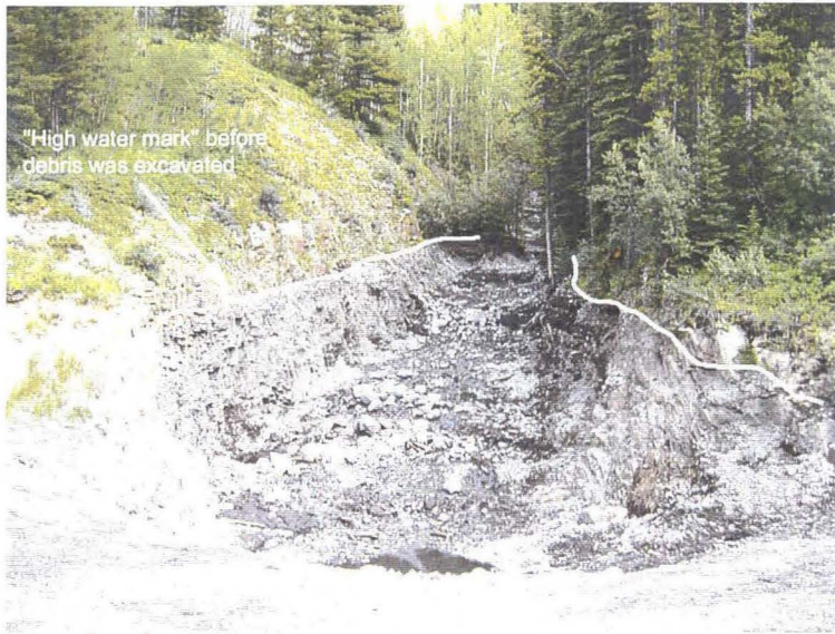
Photo 1 (top) – Facing upstream along the Hood Creek channel from Highway 40. It is understood that prior to the site inspection in July 2005, the highway maintenance contractor removed a significant volume of debris that had accumulated in the channel and blocked the culvert. Note the “bathtub ring” effect showing the high water mark from before the debris was cleared. It appeared that debris had been excavated from along the channel for a distance of approximately 80 m upstream of the highway and that around the culvert inlet the thickness of debris that was excavated was in the order of 5 to 6 m. It is not known if the debris was deposited during a single event or had built up over multiple years.
