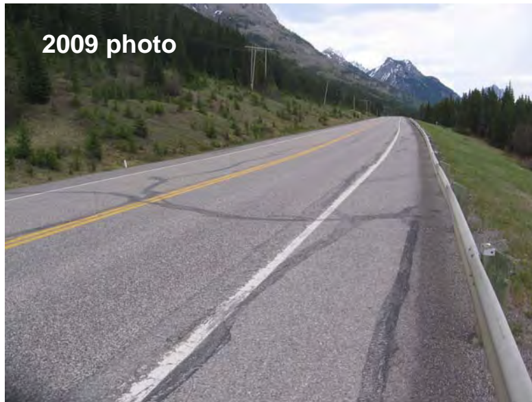
Photo 3 (top) – June 2009 Fortress Junction Road Cracking Site Facing southbound across the settlement and cracking area in the southbound lane. The pattern of the cracking and downdrop is suggestive of slumping of a segment of the downslope lane, however when compared to Photo 4 from the 2005 inspection it does not appear that the damage to the road surface has worsened in recent years.
