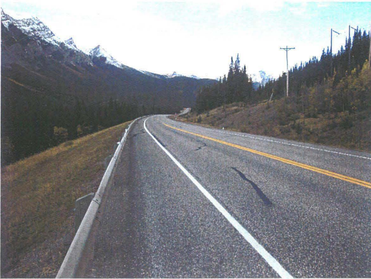
Photo 2 (bottom) – Facing north across the same area shown in Photo 1. The potential slumping affects the southbound lane and encroaches slightly into the northbound lane.
