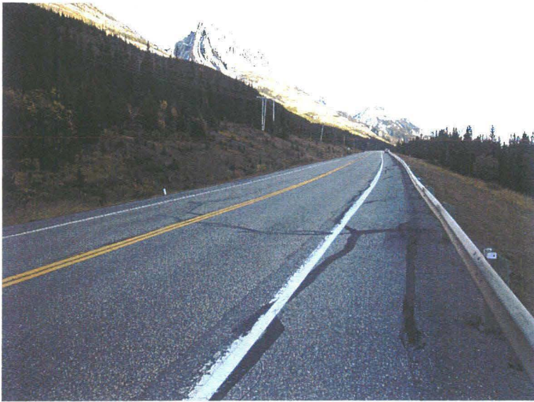
Photo 1 (top) – Facing south along the settlement and cracking area in the southbound lane of Highway 40, approximately 1 km south of the Fortress Junction service station. The cracks are in a circular pattern suggesting slumping of the southbound lane to the west (i.e. down to the right, as seen in this photo). The cracks have been sealed by the maintenance contractor. It is not known when the cracks formed or if the slumping is active. The vertical dropdown of the southbound lane to the west of the cracks varied up to a maximum of 25 mm at the time of the inspection.
