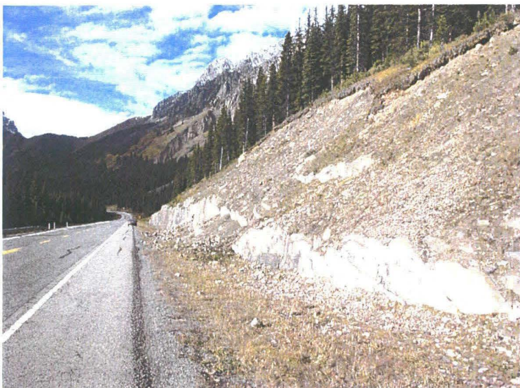
Photo 2 (middle) – Facing north along the ditch. The rockfall debris from the cut slope is contained within the ditch. As the volume of debris in the ditch builds up, some of the larger rocks roll closer to the edge of the pavement. At the time of the September 2005 inspection there were some cobble-sized rocks within 1 m of the edge of the pavement.
