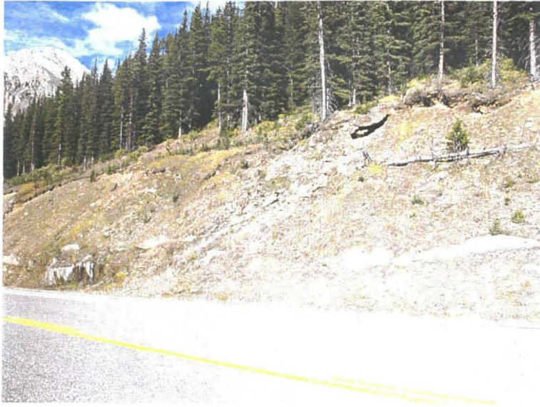
Photo 4 (top) – Another view of the cut slope slumping shown in Photo 3.
