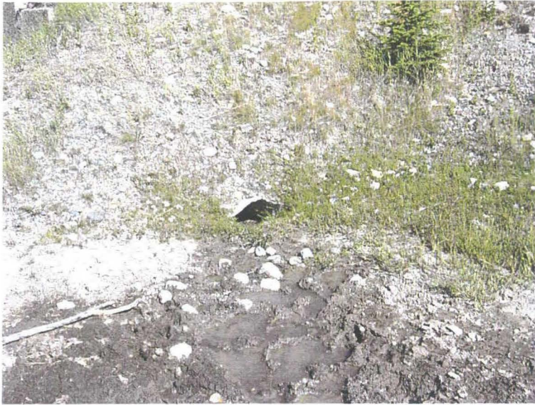
Photo 4 (top) – July 2005 – Inlet of the culvert adjacent to the east end of the wall and largely blocked by soil deposited in the ditch below an erosion area on the slope above the road (just east of the retaining wall and as shown on Photo 3).
