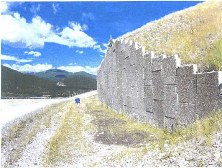
Photo 1 (top) – July 2005 – Facing west along the eastern end of the retaining wall above the road. The maximum height of this wall was approximately 6 to 7 m. There is a distinct visual appearance that this wall is leaning outwards. However, it is not known if any tilting of the wall towards the road occurred during or shortly after construction as the retaining strips behind the wall were loaded for the first time or if ongoing tilting of the wall is occurring.
