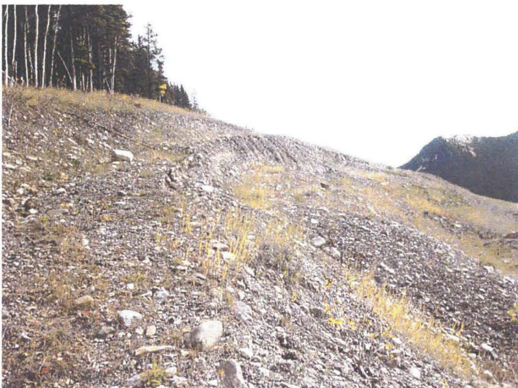
Photo 2 (middle) – Facing east along one of the visible slump scarps near the crest of the cut slope above the road. The slump scarp and vertical dropdown of the slump block is well-defined in the slope profile, however the overall visual appearance does not indicate recent significant movement of the slump block.
