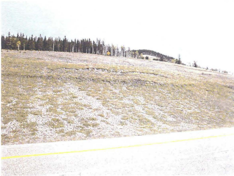
Photo 1 (top) – Cut slope above the highway. Total height estimated to be 25 to 30 m and the crest-to-toe slope angle is approximately 21°. There are numerous arcuate slump scarps in the cut slope with vertical dropdowns typically ranging between 0.5 and 1.5 m. The slump scarps often coincide with areas of seepage discharge on the slope. There appears to be little to no impact to the ditch or northbound lane of the highway from the slumping.
