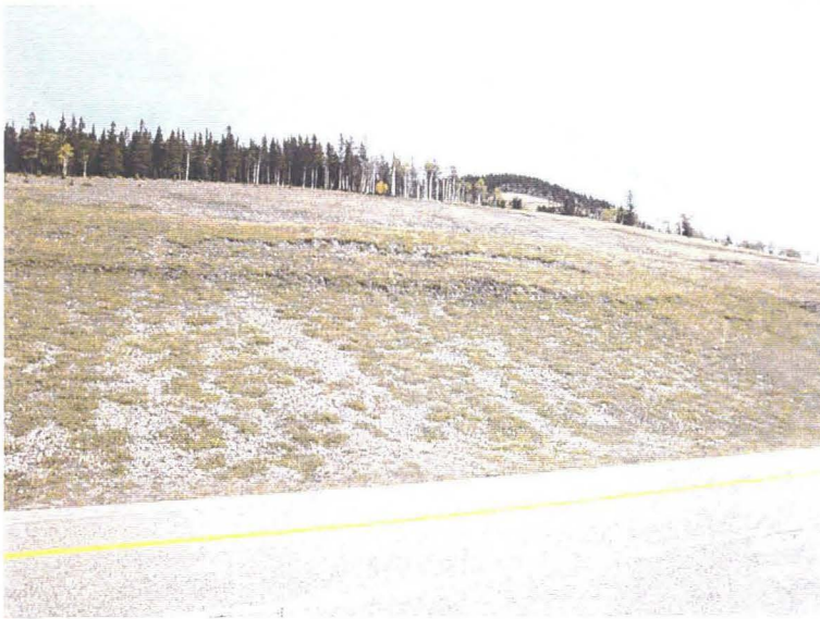
Photo 1 (top) – Cut slope above the highway. Total height estimated to be 25 to 30 m and the crest-to-toe slope angle is approximately 21°. There are numerous arcuate slump scarps in the cut slope with vertical dropdowns typically ranging between 0.5 and 1.5 m. The slump scarps often coincide with areas of seepage discharge on the slope. There appears to be little to no impact to the ditch or northbound lane of the highway from the slumping.
