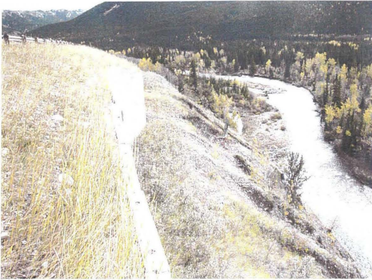
Photo 7 (top) – Eastern end of the retaining wall below the Mount Armstrong viewpoint. This view illustrates the relative position of the erosion gullies in the steep slope below the wall and the toe of the wall. The minimum offset between the toe of the wall and the head of one of the erosion gullies was approximately 3 m. Some short lengths of metal strips used in retaining wall backfill were exposed in one of these gully heads, however it is not clear if these strips were waste material from when the wall was constructed or if they had been placed in an attempt to stabilize the soil around the head of the gully.
