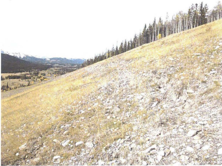
Photo 4 (top) – Facing west across the lower to middle portions of the cut slope above the highway. A slump scarp is visible in the right foreground of the photo. A number of similar scarps were noted at various locations on the cut slope, however they generally did not appear to have experienced significant movement in recent years.
