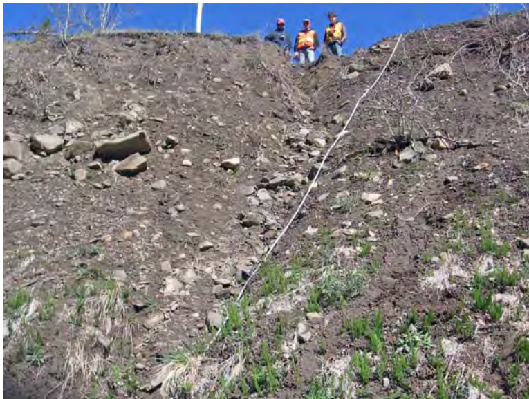
Photo 4 – June 2009 The erosion gully from near the creek level.
