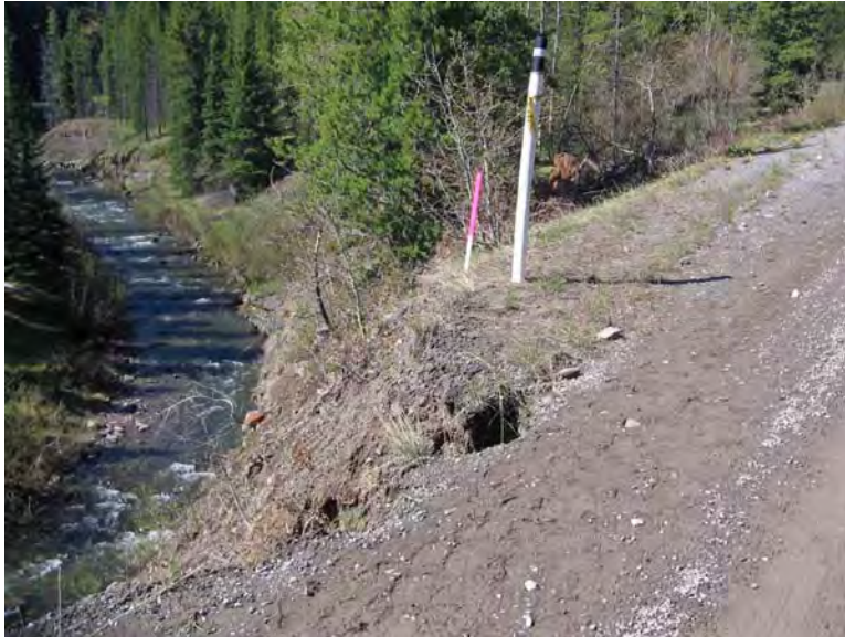
Photo 3 – June 2009 Another view of the erosion gully encroaching onto the road surface.
