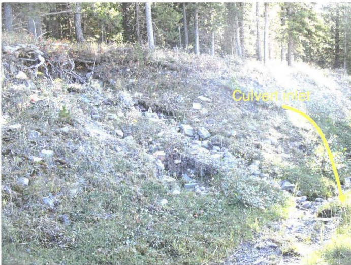
Photo 940-5 (bottom) – Secondary (south) fork of the seasonal creek in the slope above the highway, draining directly towards the culvert inlet.
