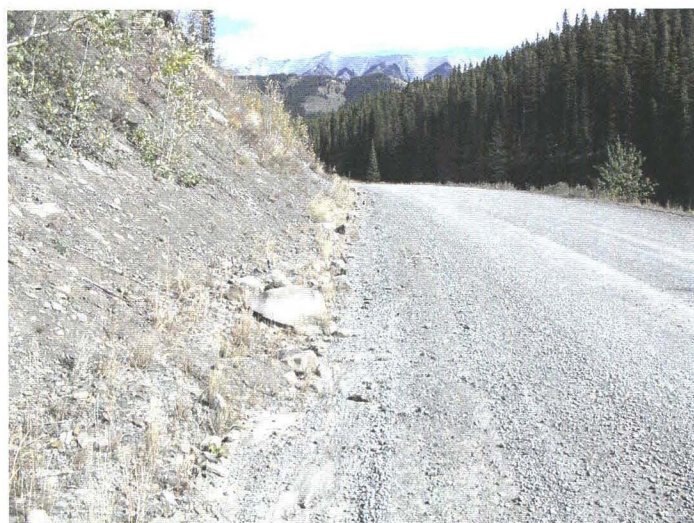
Photo 940-29 (bottom) – A boulder-sized rock that has been eroded from the cut slope and come to rest along the edge of the highway.
