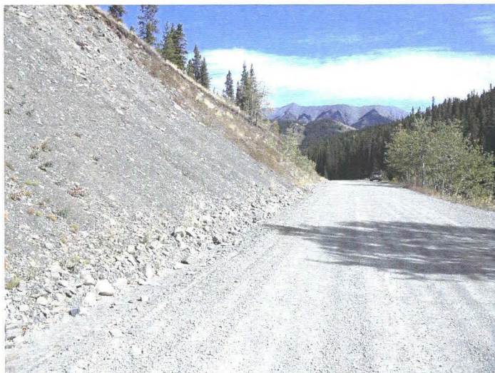
Photo 940-28 (middle) – Closer view facing east/northbound. Note the lack of a ditch and the accumulation of material eroded from the cut slope along the upslope side of the road.
