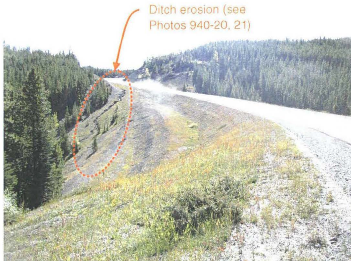
Photo 940-19 (top) – Facing southbound across the downstream embankment slope. Note the benched embankment slope. Also note the erosion visible along the segment of the east road ditch between the upland area south of the creek valley and the creek channel.
