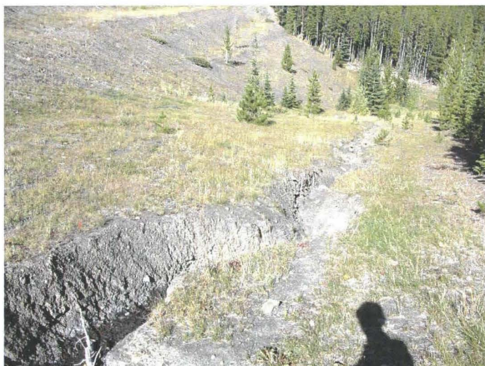
Photo 940-21 (bottom) – Facing downstream along the eroded segment of the east road ditch (same area as shown in Photo 940-20).
