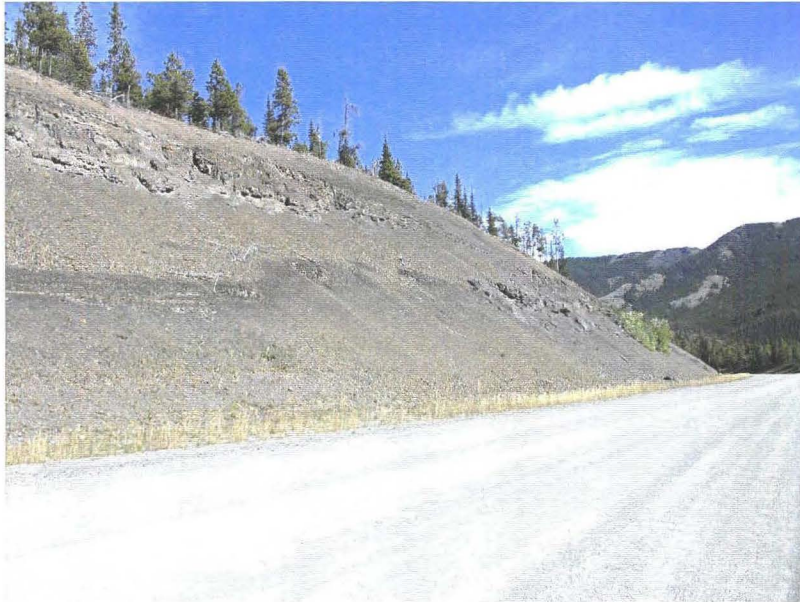
Photo 940-15 (top) – Facing northbound across the Km 20.2 Cut Slope site. The mid-slope bench retains debris from the near-vertical uppermost portion of the rock cut.
