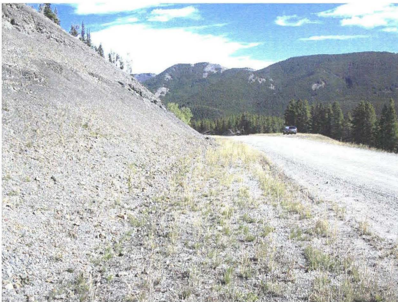
Photo 940-18 (bottom) – Facing southbound along the ditch at the Km 20.2 Cut Slope site. Note the debris accumulation into the upslope side of the ditch.
