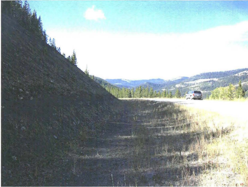
Photo 940-13 (top) – Facing northbound along the ditch adjacent to the cut slope. The shadow on the cut slope mostly obscures the weak bedrock that is exposed in the cut. This bedrock weathers into gravel-sized pieces of dark grey shale and fine grained soil.
