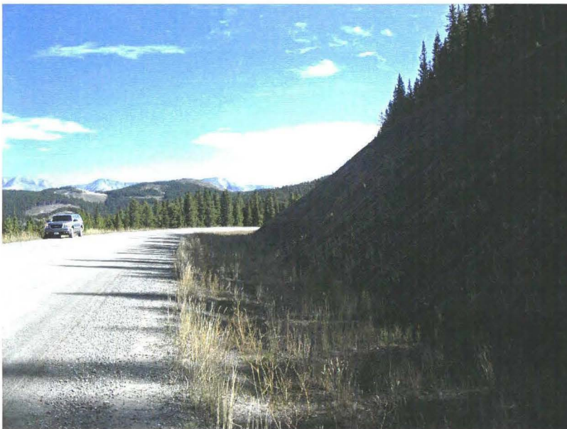
Photo 940-14 (bottom) – Facing southbound along the ditch adjacent to the cut slope.
