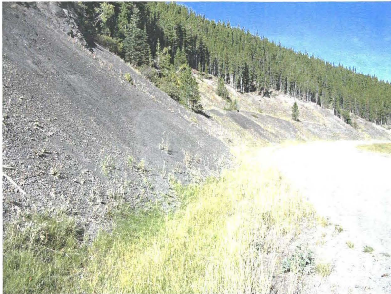
Photo 940-11 (top) – Facing northbound along the ditch, with debris encroaching into the ditch base visible.
