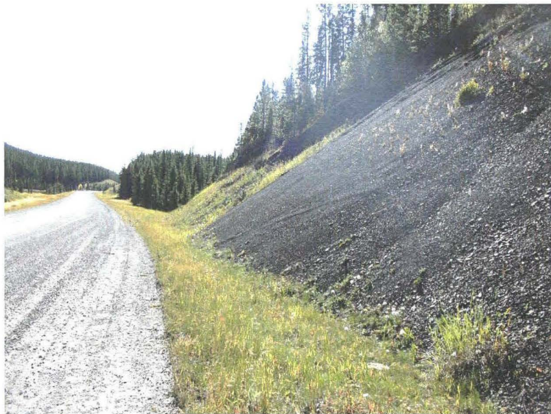
Photo 940-12 (bottom) – Facing southbound along the ditch, with debris encroaching into the ditch base visible. At the time of the inspection, only a few of the gravel-sized pieces of debris had rolled beyond the ditch and onto the road surface.
