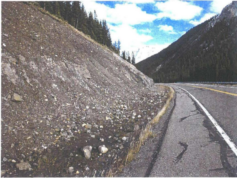
Photo 1 (top) – Facing southeast across the site. The northern end of the cut slope (visible in the foreground) exposes rocky soil at an angle of 45^\circ overlying a rock cut at about 60^\circ . Gullying of the exposed soil has released cobble to boulder-sized rocks and an apron of this debris has built up along the toe of this segment of the cut slope. Cobble to boulder-sized material has been deposited within 2 m of the edge of the pavement. The thickness of the exposed soil in the upper portion of the cut slope tapers out towards the southeast. The southeast end of the cut slope (in the background of this photo) exposes intact bedrock at an overall angle of 45^\circ with very little debris in the ditch below.
