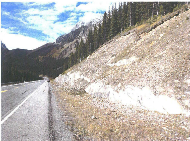
Photo 2 (middle) – Facing north along the ditch. The rockfall debris from the cut slope is contained within the ditch. As the volume of debris in the ditch builds up, some of the larger rocks roll closer to the edge of the pavement. At the time of the September 2005 inspection there were some cobble-sized rocks within 1 m of the edge of the pavement.
