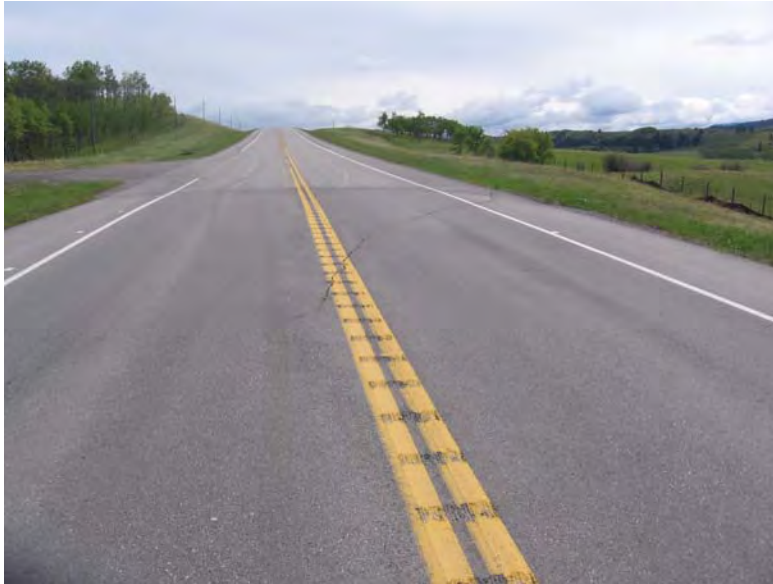
Photo S16-1 (top) – June 2009 Facing south across the southern end of the repair area that was repaved in early 2007. The crack across the southbound lane remains visible, and has not changed significantly since it formed during 2007.
