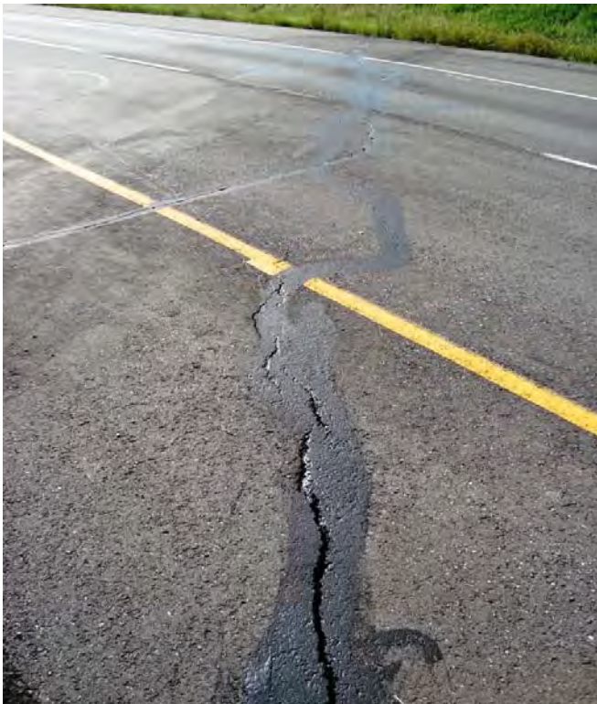
Photo S25-3 – June 2012 Facing southeast across the eastbound lane at the cracking in the easternmost patch. The cracking here had approximately 20 mm aperture with no down-drop and may be indicative of active sliding in this area.
