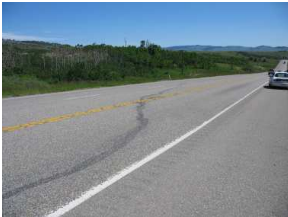
Photo S27-3– June 2007 (lower left) Closer view, facing east, of the east end of the cracking area. At the time of the June 2007 site inspection the portion of the highway to the east of the crack was subtly downdropped relative to the west.
