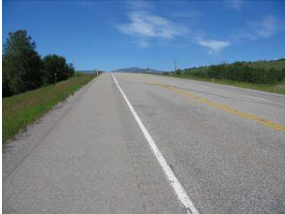
Photo S27-1– June 2007 (upper left) Facing west along the highway with the diagonal crack visible across the entire road width.
