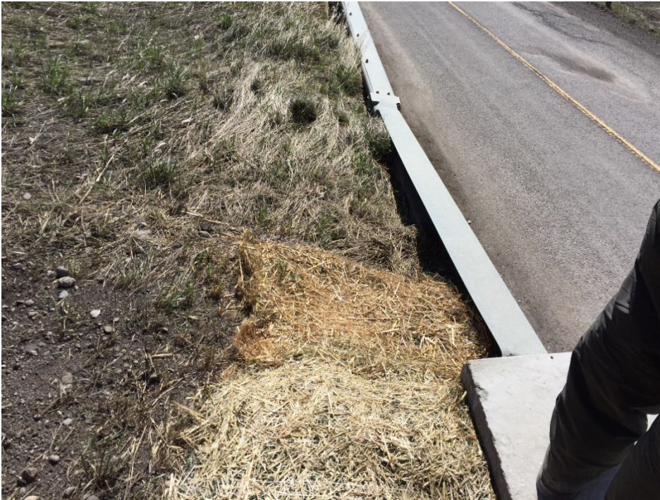
Photo 3 Transition area from new concrete retaining wall to existing steel bin wall. Small voids still remain.
