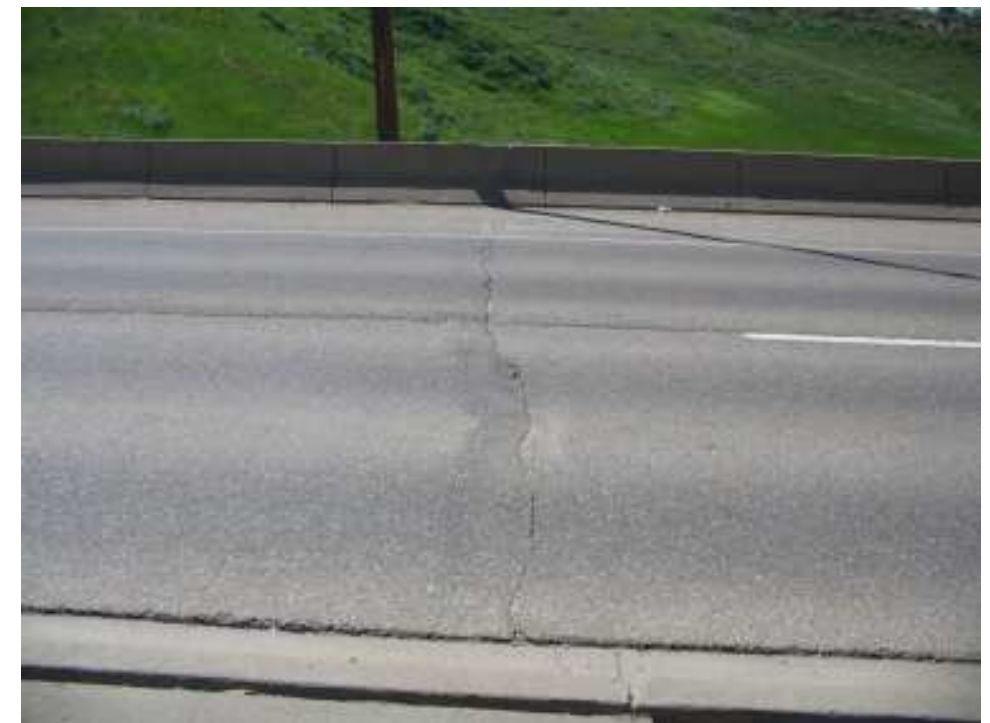
Photo S29-6– June 2007 (lower right) An old crack perpendicular to the eastbound lanes and in the same general area as the more well-defined cracking in the westbound lanes.
