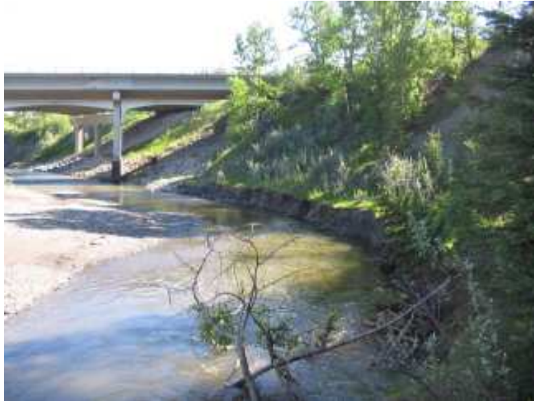
Photo S1-1 – June 2008 (top) Facing downstream along the right (east) creek bank, towards the east abutment of the eastbound lane bridge. Note the pronounced bank erosion visible where peak flows in the east creek sub-channel have created a 1 to 1.5 m high, near-vertical soil bank. It appears that segments of the east bank have eroded up to 1 to 2 m in the past couple of years.
