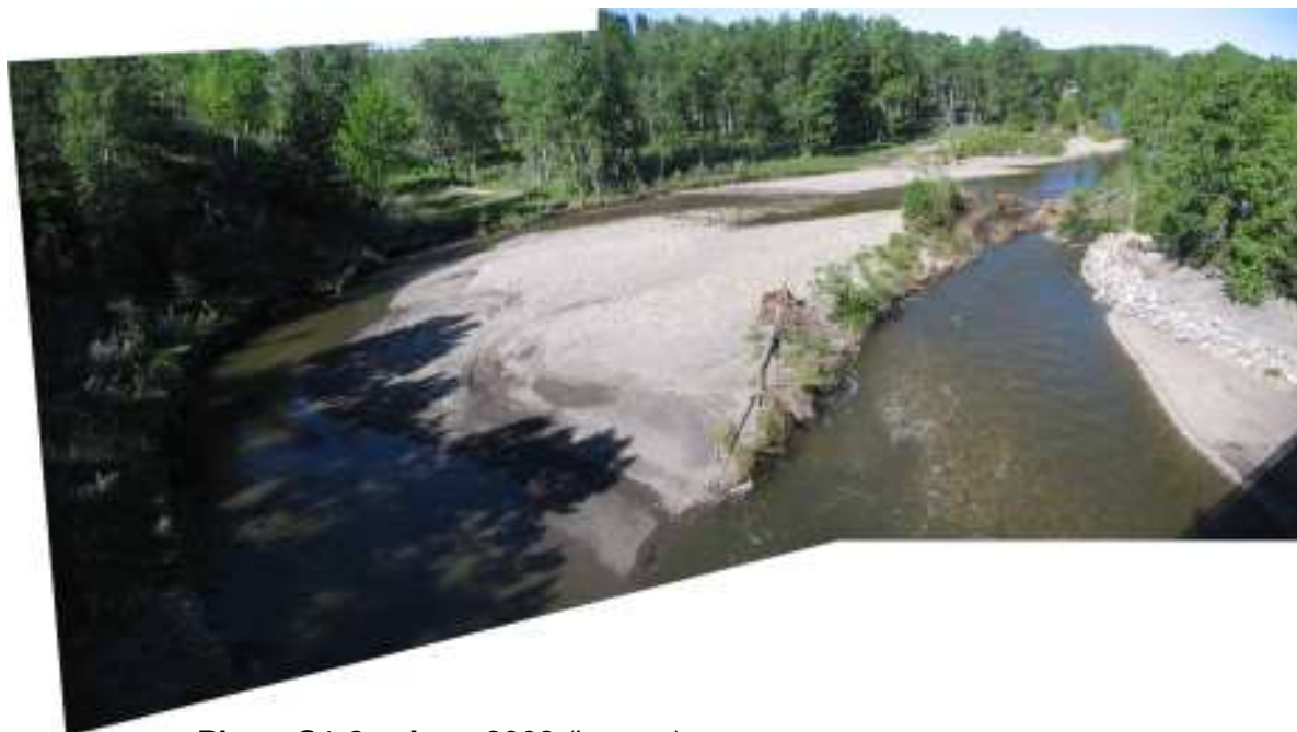
Photo S1-2 – June 2008 (bottom) Facing upstream from the middle of the eastbound lane bridge deck. The west sub-channel (on the right hand side of the photo) appeared to be carrying the majority of the flow at the time of the inspection. It appeared that earlier peak flows in the east sub-channel (left on photo, largely in shadow) had recently eroded significant volumes of soil from the east bank, as shown in Photo S1-1.
