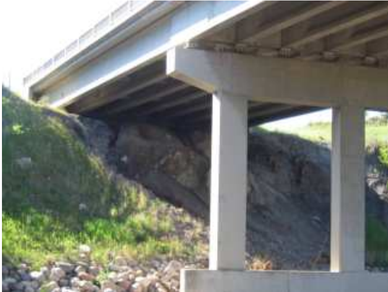
Photo S1-3 – June 2008 (top) Surface erosion and gullying of the exposed shale bedrock in the east abutment slope of the eastbound lane bridge. It appears that the erosion is caused by overflow of bridge deck runoff from the collection gutters below the east end of the bridge. The appearance of the erosion and gullying has gradually worsened over time since the annual inspections began in 2000, but did not appear to have worsened significantly since the 2007 inspection.
