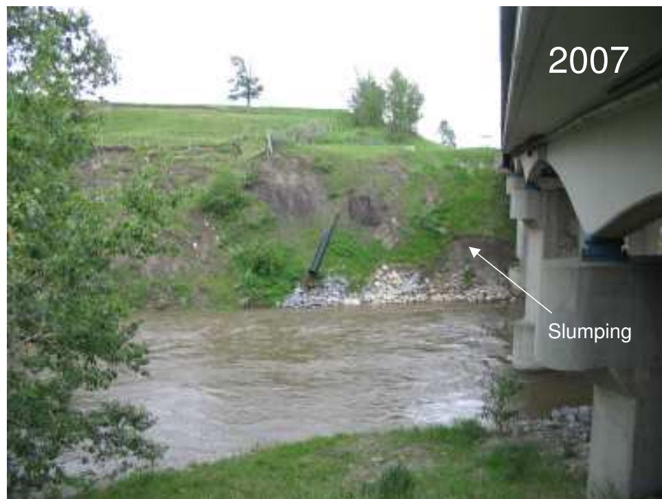
Photo S1-3 – June 2007 (lower left) East creek bank, downstream of the westbound bridge. The slumping just above the upslope limit of the rip-rap armouring appears to have increased slightly in size since the 2006 inspection (see Photo S1-4) however it does not appear to have developed into a significant risk to the bridge abutment stability to date.
