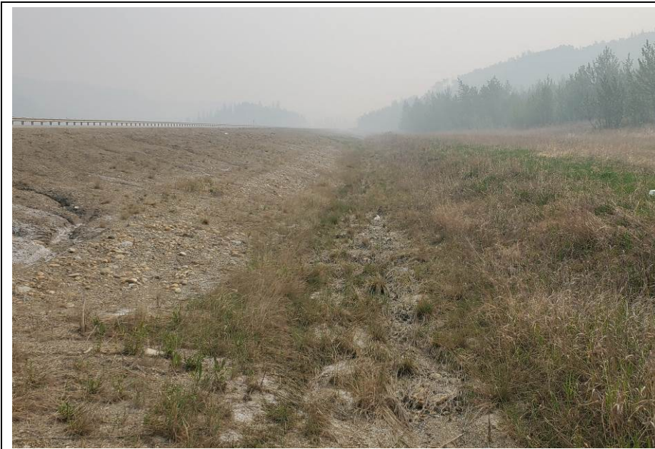
Photo 7-13. Looking upslope the ditch (east) at the gabion mattress section (32+500). Section had vegetation growth and was performing well. Minor rill damage was noted on the north side of the ditch.
