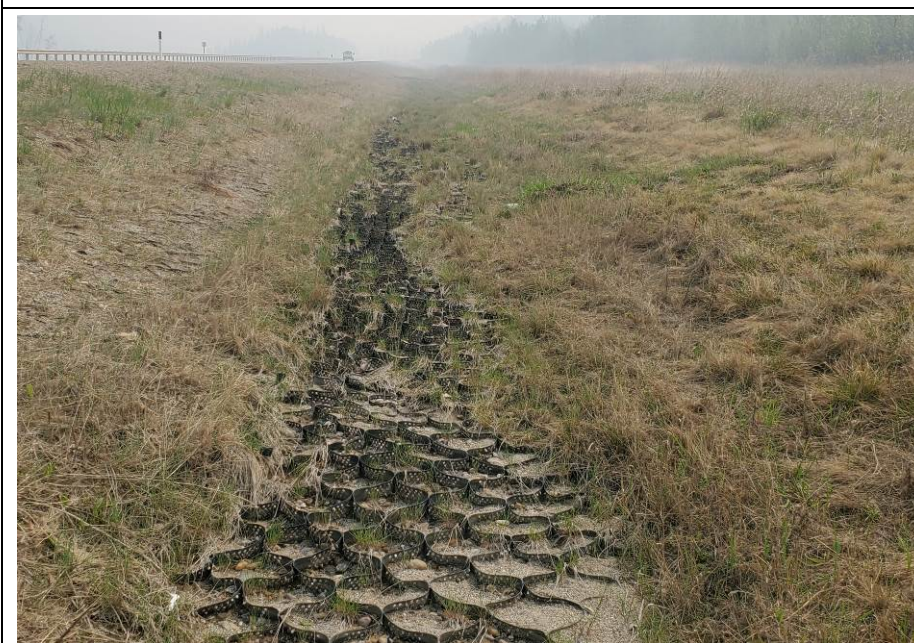
Photo 7-12. Looking upslope the ditch (east) at the geoweb control section (32+400). No major change since the 2020 condition; Section had vegetation growth and some cells were only partially filled and broken. Some minor rill damage was noted on the north side of the ditch.
