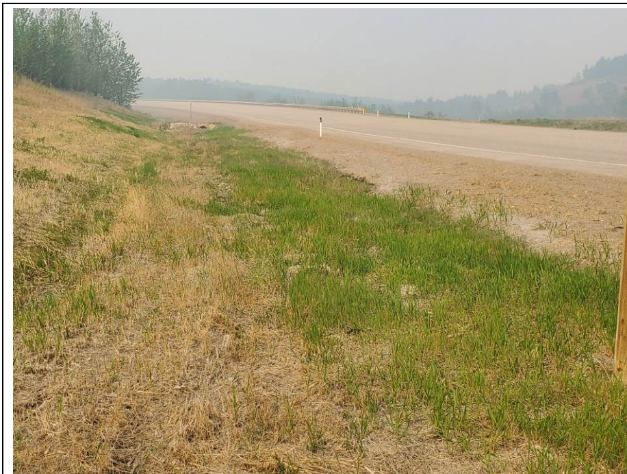
Photo 7-09. Previously observed channelized erosion has since revegetated on the north side of the ditch within the rolled erosion control product (turf reinforced matting) test section (32+100).
