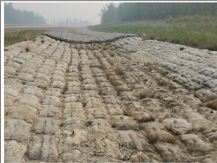
Photo 7-17. Looking east (upslope) at the top of the erosion control test ditch (32+900). Ditch upslope of the test section has been lined with gabion mattress as part of the 2018/2019 East Daishowa (PH42) mitigation work. The ditch and new mitigation works were in good condition with no observable change from the 2020 condition.
