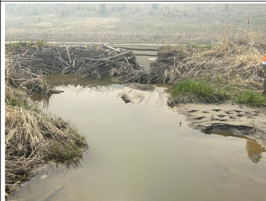
Photo 7-02. Maintenance contractor excavated a drain slot through beaver dam to drain water into the channel near km 32+825.
