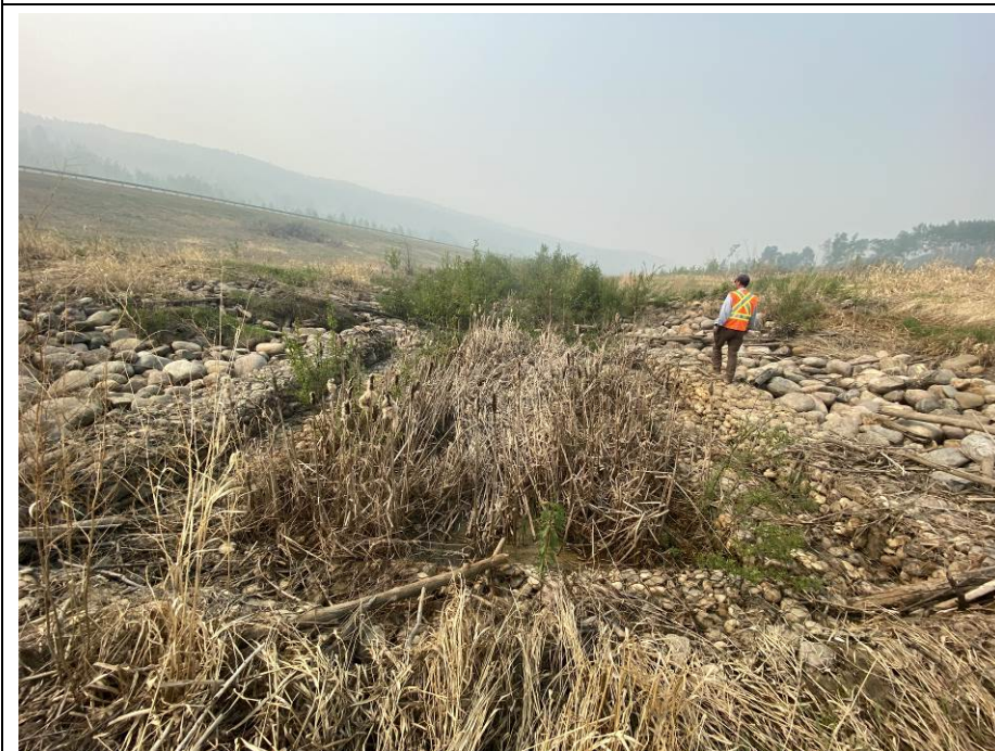
Photo 7-06. North channel gabion inlet structure. Cat tails growing within centre of channel, but flow capacity is still ok. Condition was generally comparable to previous inspections (32+855).
