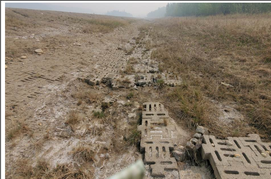
Photo 7-14. View of the damage within the interlocked concrete block (i.e. Lafarge paving stones) paving stone section (32+600). Blocks have deteriorated and broken up in numerous locations and have been undermined by erosion exposing geotextile fabric beneath. Overall section is worse relative to the other test sections.
