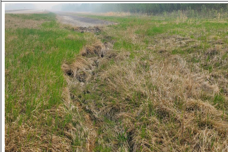
Photo 7-10. Looking east towards 300 m diameter channel sock erosion control section (32+150). Section had good vegetation growth through area of previous channelized erosion near the downstream boundary of the geomembrane section.
