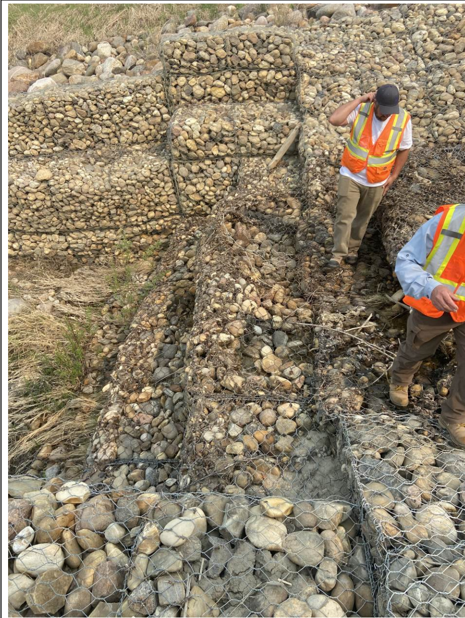
Photo 7-04. Close-up view of the internal upper gabion drop structure (32+540). Baskets in the channel centre have some bagging and broken wire. Maintenance is recommended to prevent further damage / loss of gabion rock. Overall, the structure is intact and functioning as intended.
