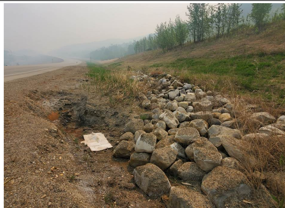
Photo 7-08. Erosion around the culvert intake structure at the west end of the erosion control test ditch (32+050). Erosion has slightly filled in since the 2020 condition but area still needs to be graded and riprap adjusted to ensure water flow enters the culvert.
