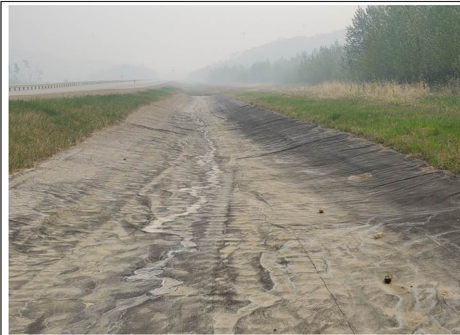
Photo 7-11. Looking upslope (east) at the Coletanche geomembrane erosion control section (32+250). Was in good condition with no new damage observed in previous patch repair area.
