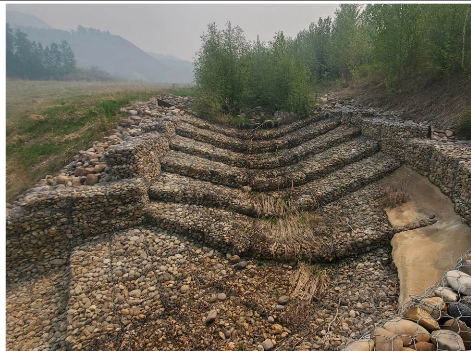
Photo 7-07. View of the upper segment of the gabion channel bend and drop structure (31+800). Gabions within the middle of the channel showing some bagging and wire damage that will require eventual maintenance to prevent further basket damage. Overall structure was intact and functioning as intended.
