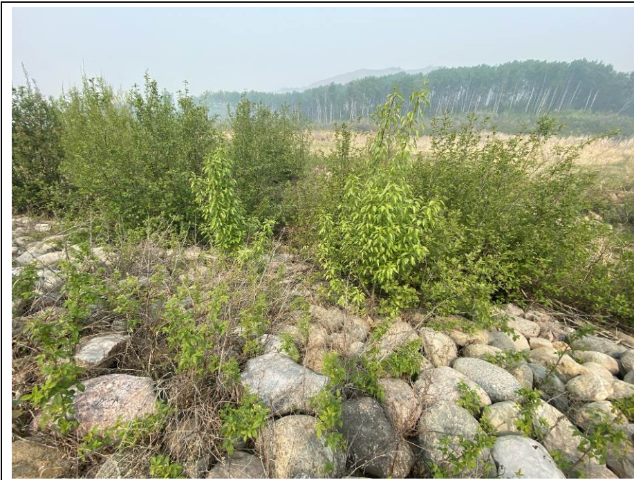
Photo 7-03. Alder and willow tree growth within the riprap downstream of the armoured channel inlet near km 32+800.
