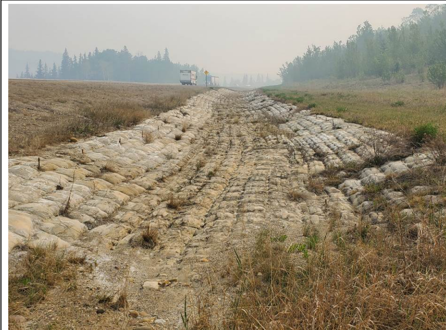
Photo 7-16. Looking east towards pillow concrete section (32+800). Section was performing well. Minor concrete deterioration was noted in select areas, but erosion mitigation function was not impacted.
