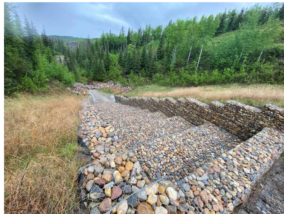
Photo 43-12. Site B- view northeast from the top of the gabion drop structure the culvert outlet in the valley bottom (33+600). Top of structure appeared in good condition with no major change from the 2023 condition.
