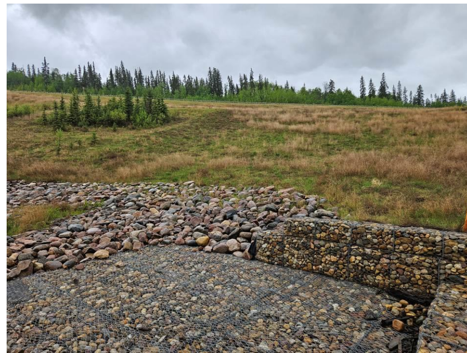
Photo 43-04. Looking south at the area of previous slumping associated with culvert erosion below pile wall and regraded slide during construction in 2017 (33+430). Area has since revegetated following grading of the construction access. No change from 2023 condition.
