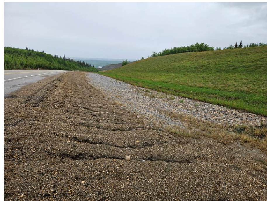
Photo 43-20. Rill erosion between the road and north ditch gabion armour (km 34+000) was slightly worse compared to the 2023 condition. TRM should be added to reduce rates of erosion.
