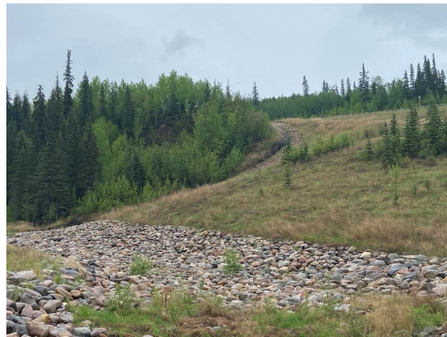
Photo 43-05. Site A - Standing at the top of the gabion drop structure looking southeast towards the rock washout and gully erosion in the armoured swale near 33+525. Erosion was worse from 2023. Armoured overflow channel in the valley bottom was in good condition.
