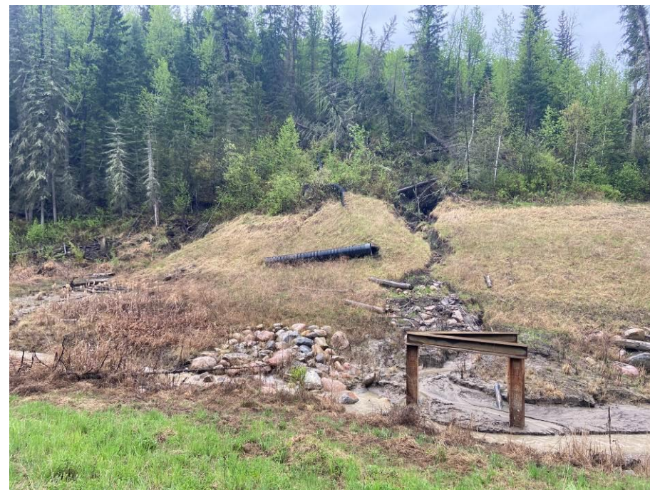
Photo 43-16. Looking south towards the outlet of the CPP down pipe near the culvert inlet (33+850). Gully erosion was noted to be occurring upslope from the pipe outlet due to a leaking joint that requires repair. Increased gully erosion was noted on the right side of the pipe. Large gully erosion headwall developing upslope in the trees and sliding of gully sidewalls. Expanded erosion since 2023.
