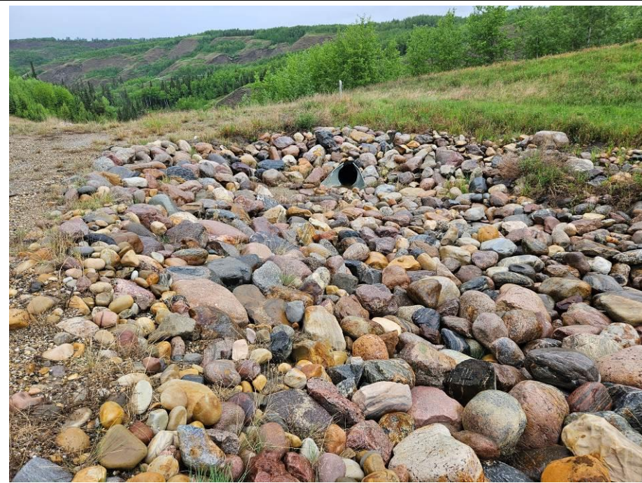
Photo 43-18. View of culvert inlet and riprap protection near 33+900 on north side of road. No visible changes from the 2023 condition.
