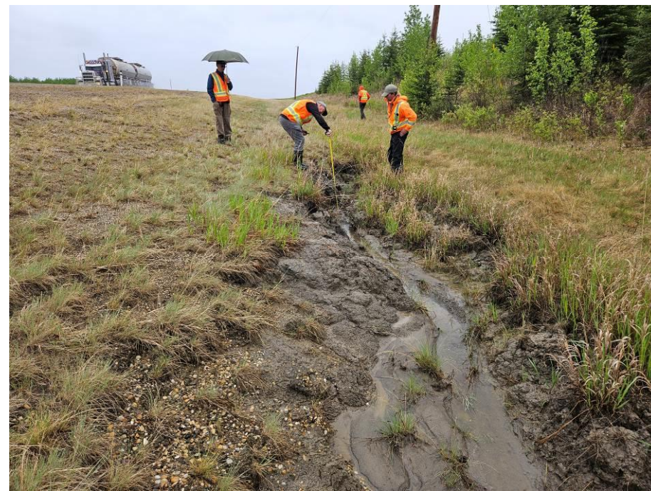
Photo 43-19. Looking upslope (east) at the south ditch erosion where a gully has developed (up to 1.2 m wide, 0.7 m deep) between approximately 33+900 and 34+150. Erosion has become deeper and wider since 2023.
