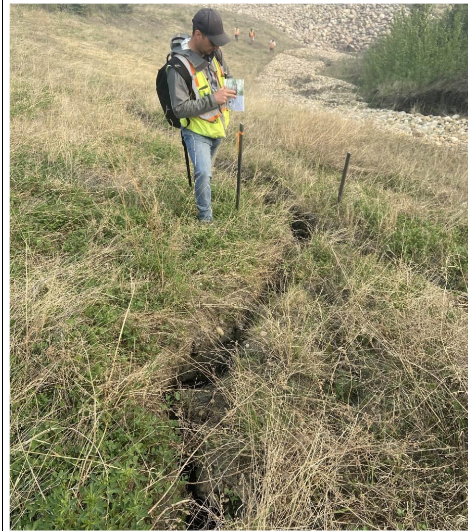
Photo 43-08. Looking towards the north at survey lath stakes installed in 2023 to monitor a potential tension crack related to potential downslope movement towards the swale washout and erosion area (km 33+500). The offset between the outside base of the stakes measured 1.16 m and did not increase relative to the previous measurement. Feature could be result of erosion.
