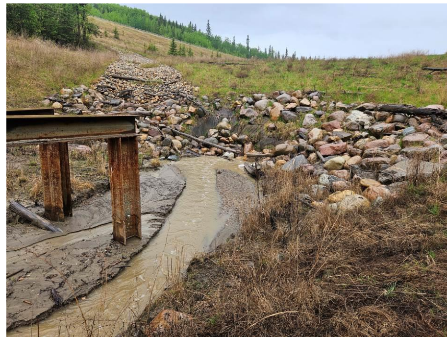
Photo 43-15. Damage around culvert inlet due to a high flow event in 2021/2022. Culvert pipe at the inlet was effectively pinched and twisted shut and was filled with woody debris. Additional riprap above the inlet has collapsed and buried it. Additional woody debris buildup. Repairs required in this area (33+800).
