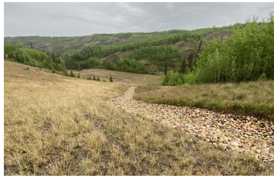
Photo 43-17. Looking northwest from the top of Site B towards the armored swale and overland flow area (33+875). No changes from the 2023 condition.
