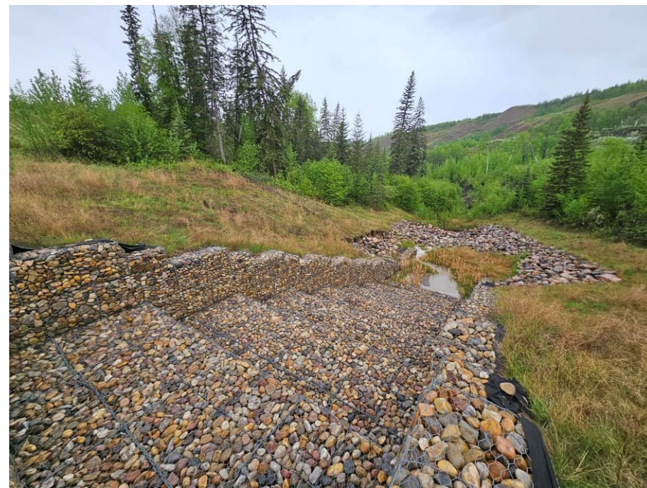
Photo 43-03. Overflow gabion drop structure and dissipation bowl at the previous culvert outlet that had extensive erosion and gulying below Site A (33+430). Some rill erosion was noted within the fill areas that were still vegetating. Dissipation bowl at base of drop structure had a large amount of silt buildup. Minor change from 2023 condition.
