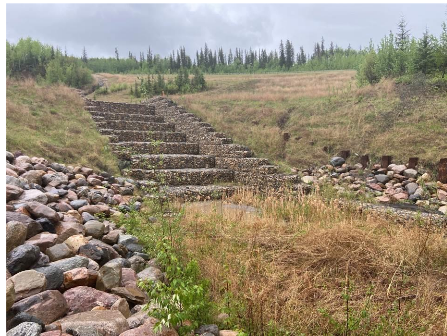
Photo 43-01. Looking towards the southeast (upstream) at the Site A gabion drop structure. No major change from 2023 condition. Rill erosion on the right side of the photo above the steel pile wall was slightly worse.
