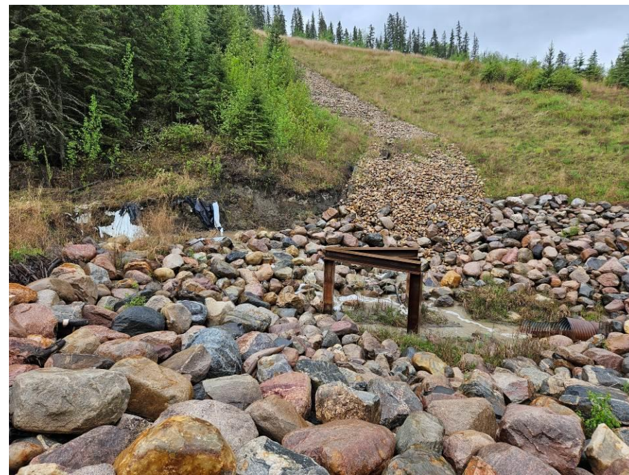
Photo 43-06. Site A - Looking south towards the culvert inlet riprap, riprap swale, and debris deflector (33+500). Note south channel bank erosion and fallen riprap. Slightly worse from the 2023 condition. Culvert inlet was damaged and eroded, causing water to flow under the base and come in at a joint.
