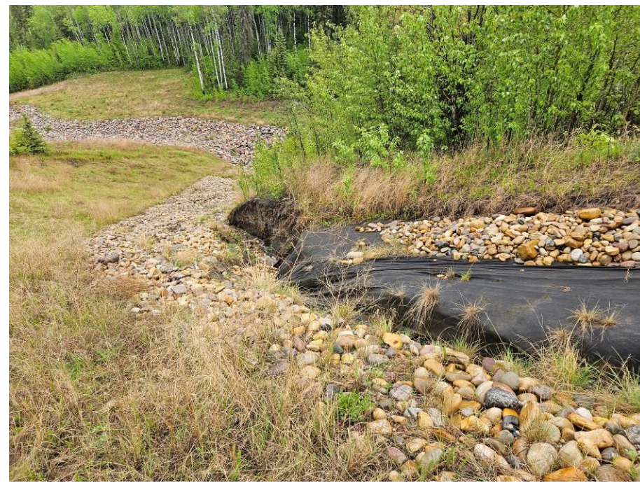
Photo 43-07. Site A - looking north, downslope towards washed out riprap and extensive erosion damage within the riprap swale at the east side of Site A (33+500), likely the result of a high-flow event in 2019/2020. Deeper and expanded erosion damage since 2023.
