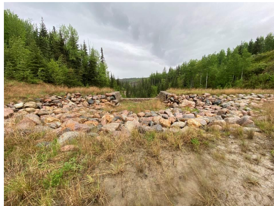
Photo 43-13. Site B- view east at upstream of the gabion drop structure with riprap berm at west end of overland flow toe berm (33+625). No change from 2023 condition.
