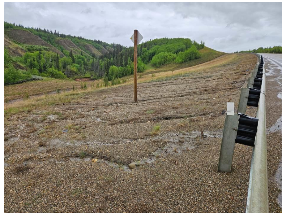
Photo 43-09. Looking east from the top of the Site B highway embankment. Minor rill erosion within top of embankment where TRM ends. No significant change from the 2023 condition.
