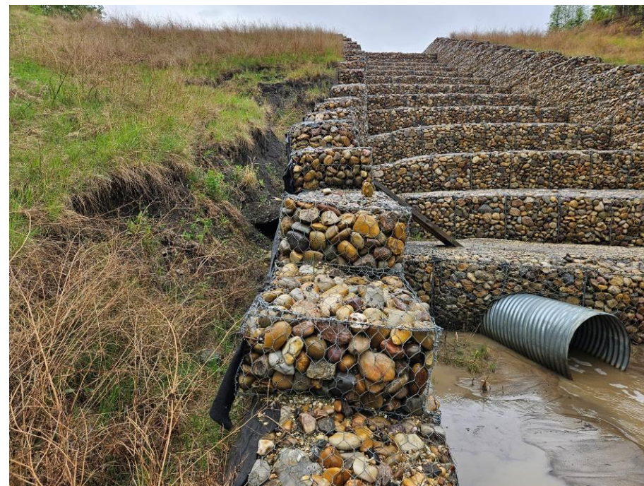
Photo 43-10. Site B- view east from the base of the gabion drop structure and riprap dissipation bowl at the culvert outlet (33+600). Additional erosion expansion and gabion deformation due to piping erosion from leak in the culvert joint (left side).
