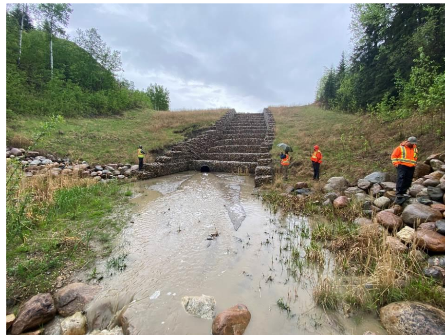
Photo 43-11. Site B- view of the gabion drop structure and riprap dissipation bowl at the culvert outlet (33+600). Additional sediment buildup in dissipation bowl.
