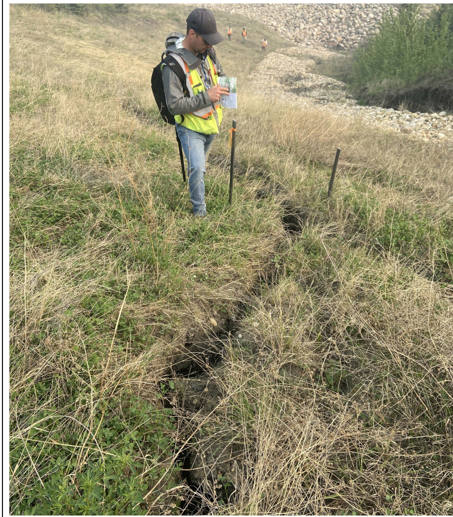
Photo 43-10. Looking towards the north at survey lath stakes installed in 2022 to monitor a tension crack related to potential downslope movement towards the swale washout and erosion area (km 33+500). The offset between the outside base of the stakes measured 1.16 m and did not increase relative to the previous measurement.
