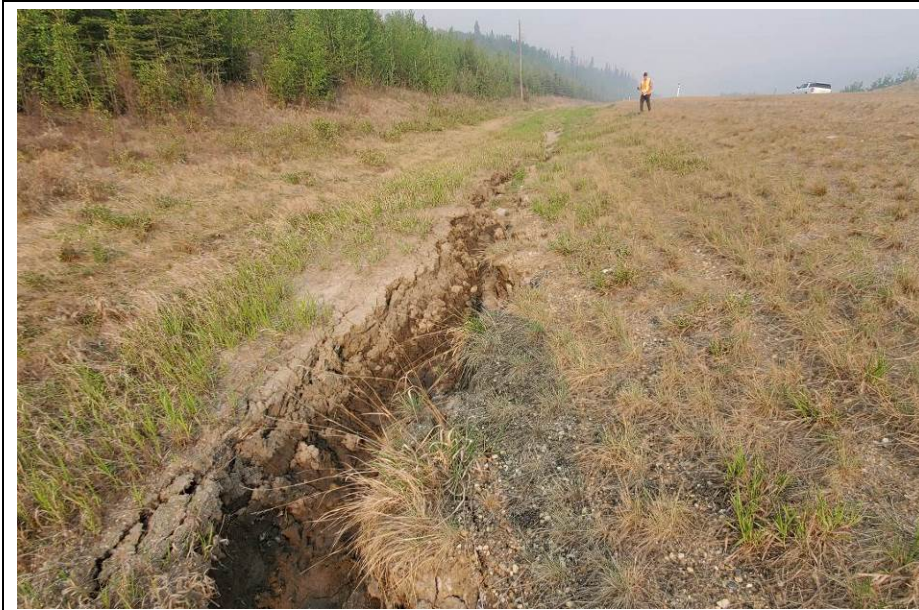
Photo 43-18. Looking west at the south ditch erosion where a gully has developed (0.8 m wide, 0.5 m deep) in area with previous erosion that had vegetated between approximately km 34+150 to km 34+000.
