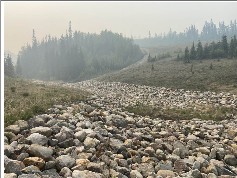
Photo 43-05. Standing at the top of the gabion drop structure looking east towards the overflow channel riprap (33+450). Vegetation has re-established.
