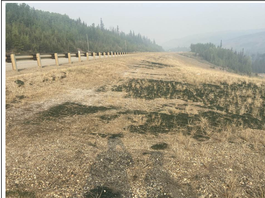
Photo 43-12. Looking west towards the TRM installation on the upper portion of the slope north of the road (33+700). Some vegetation growth has started.
