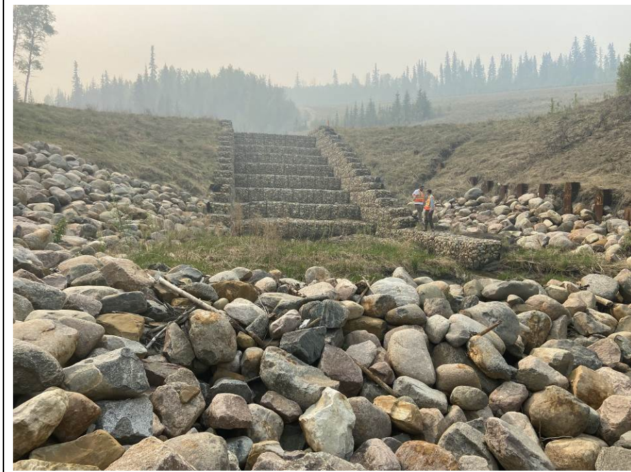
Photo 43-01. Looking towards the southeast (upstream) at the Site A gabion drop structure. No major change from 2022 condition. Rill erosion on the right side of the photo above the steel pile wall was slightly worse.
