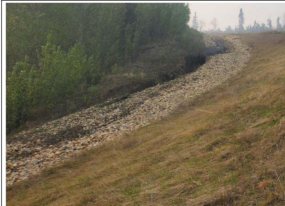
Photo 43-13. Site A - looking south, upslope towards washed out riprap and extensive erosion damage within the riprap swale at the east side of Site A (33+500), likely the result of a high-flow event in 2019/2020. Deeper and expanded erosion damage since 2022.
