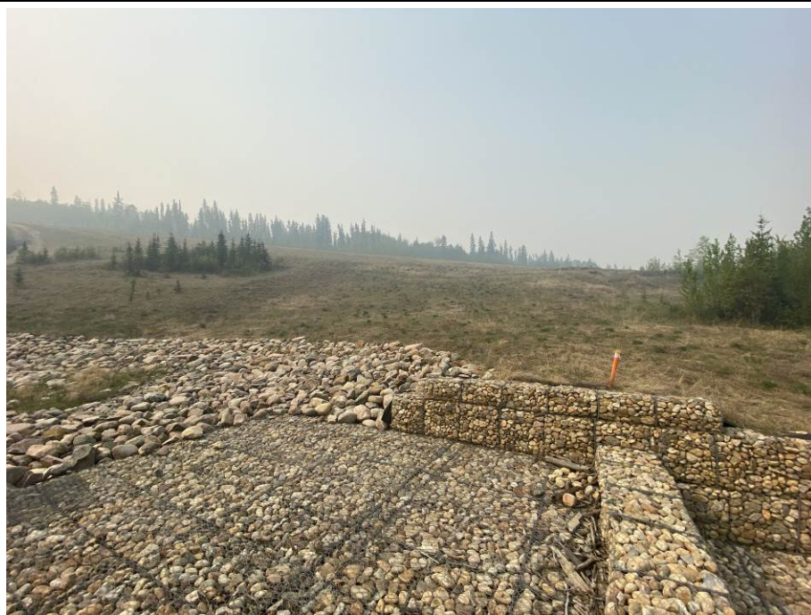
Photo 43-04. Looking south at the area of previous slumping associated with culvert erosion below pile wall (33+430). Area has since revegetated following grading of the construction access.
