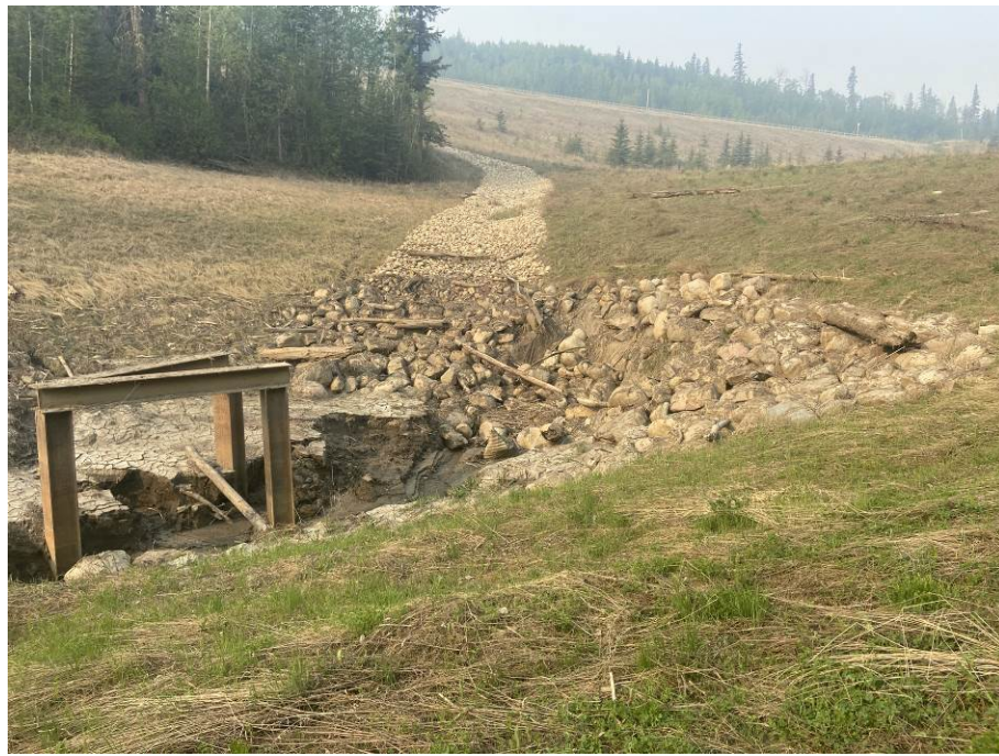
Photo 43-15. Damage around culvert inlet due to a high flow event. Culvert pipe at the inlet was effectively pinched and twisted shut and was filled with woody debris. Additional riprap above the inlet has collapsed and buried it. Additional woody debris buildup. Repairs required in this area (33+800).
