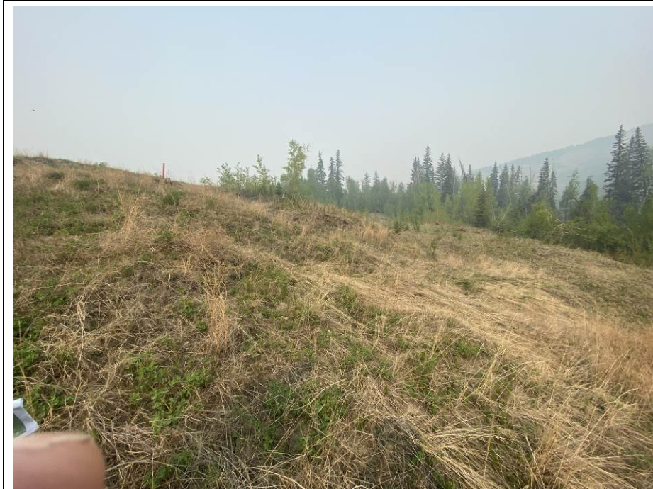
Photo 43-02. Main slide scarp of active shallow failure downslope of the buried pile wall (33+325) first observed in 2017. Area is vegetated but appears there is active movement within the disturbed slide mass.
