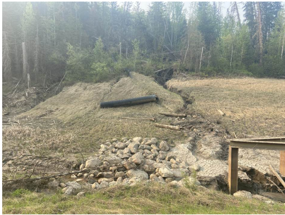
Photo 43-16. Looking south towards the outlet of the CPP down pipe near the culvert inlet (33+800). Rill erosion was noted to be occurring upslope from the pipe outlet due to a leaking joint that requires repair. Increased gully erosion was noted on the right side of the pipe.
