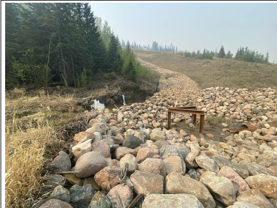
Photo 43-06. Looking south towards the culvert inlet riprap, riprap swale, and debris deflector (33+500). Note south channel bank erosion, silt buildup and erosion within the riprap swale. Slightly worse from the 2022 condition. Culvert inlet is damaged and eroded, causing water to flow under the base and come in at a joint.
