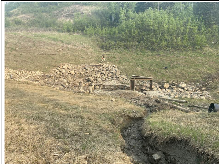
Photo 43-14. Site B culvert inlet with riprap protection and steel H-beam debris deflector. Inlet become severely damaged and blocked with fallen riprap during a high flow event in 2019/2020 (33+800). No major changes from 2022 condition. Increased erosion at gully on left side of photo. Repairs required in this area.
