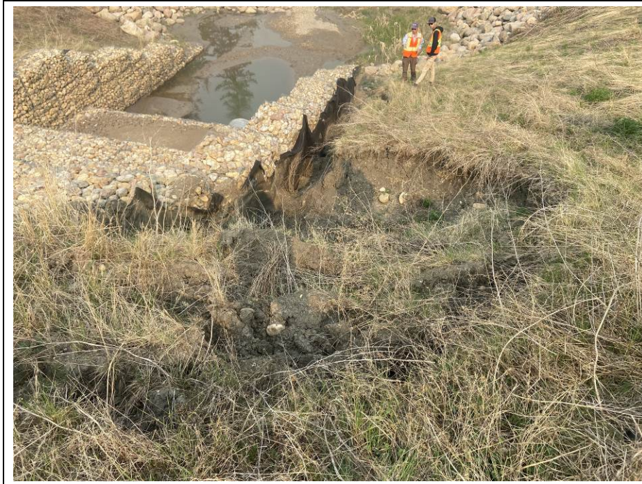
Photo 43-09. View from above of the expanded erosion and slightly worse gabion deformation due to piping erosion from leak in the culvert joint.
