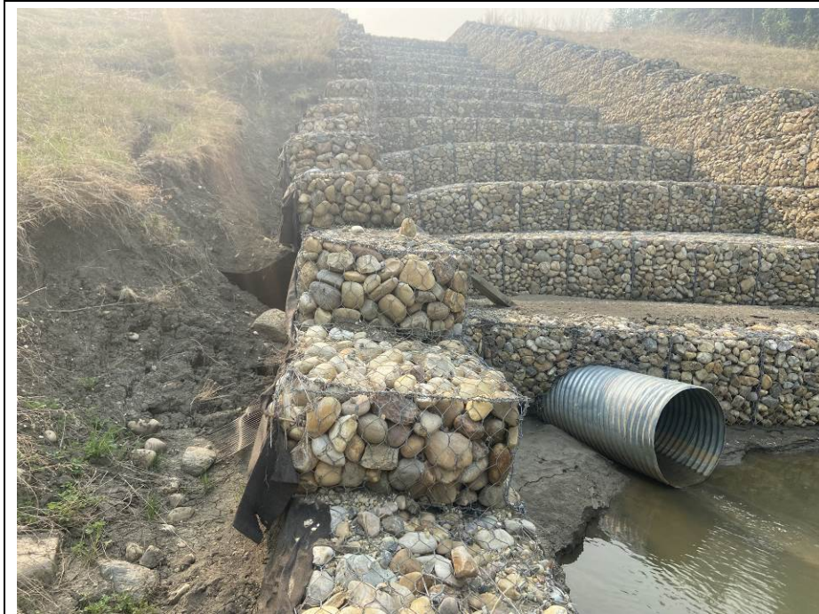
Photo 43-08. Site B- view of the gabion drop structure and riprap dissipation bowl at the culvert outlet (33+600). Additional erosion and gabion deformation due to piping erosion from leak in the culvert joint (left side).
