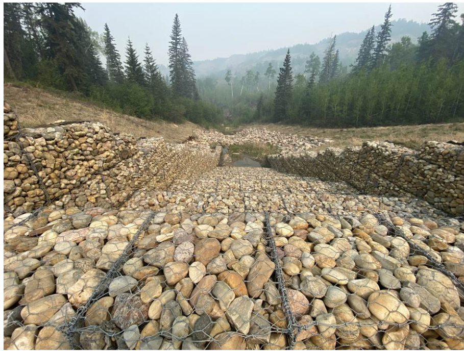
Photo 43-03. Overflow gabion drop structure and dissipation bowl at the previous culvert outlet that had extensive erosion and gullyng below Site A (33+430). Some rill erosion was noted within the fill areas that were still vegetating. Base of drop structure had a large amount of silt buildup. Minor change from 2022 condition.
