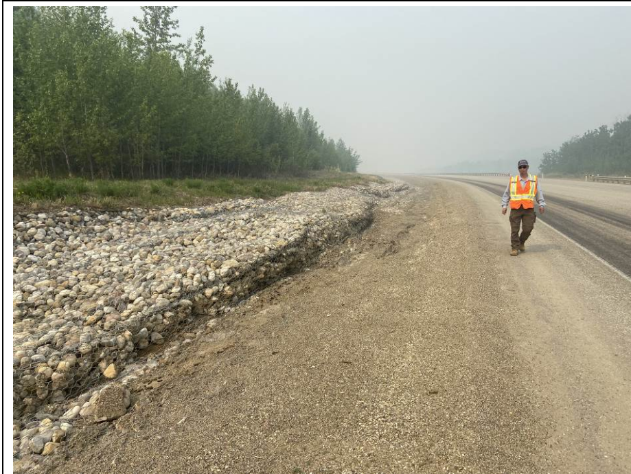
Photo 42-06. View looking west at the gabion mattress installed in the south ditch near 33+125. The toe roll of a landslide that occurred in 2020 has encompassed and deformed the gabion pushing it upwards and towards the highway. The length of gabion affected is approximately 85 m. Gabion is slightly more heaved but no significant change since previous inspection. Erosion in sideslope due to restricted flow from gabion heave.
