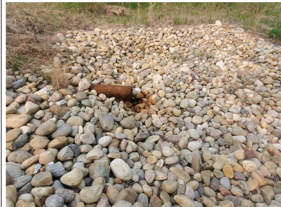
Photo 42-04. Looking at subdrain pipe outlet that was slowly dripping within the end of the armoured drainage swale from the west side of the wall.
