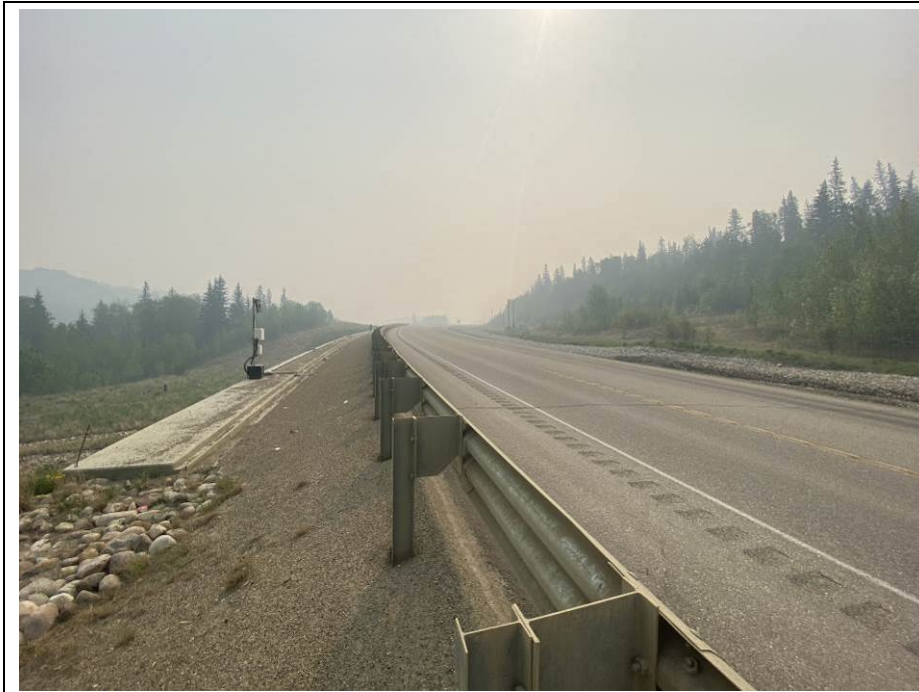
Photo 42-01. Looking east across the repaired slide area. Guardrail and pavement surface in good condition with no major change since previous inspection.
