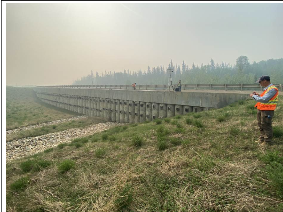
Photo 42-02. Looking southeast at the pile wall and regraded slope below. Wall appears in a good condition and there has been no observable changes in the slope below since 2021.
