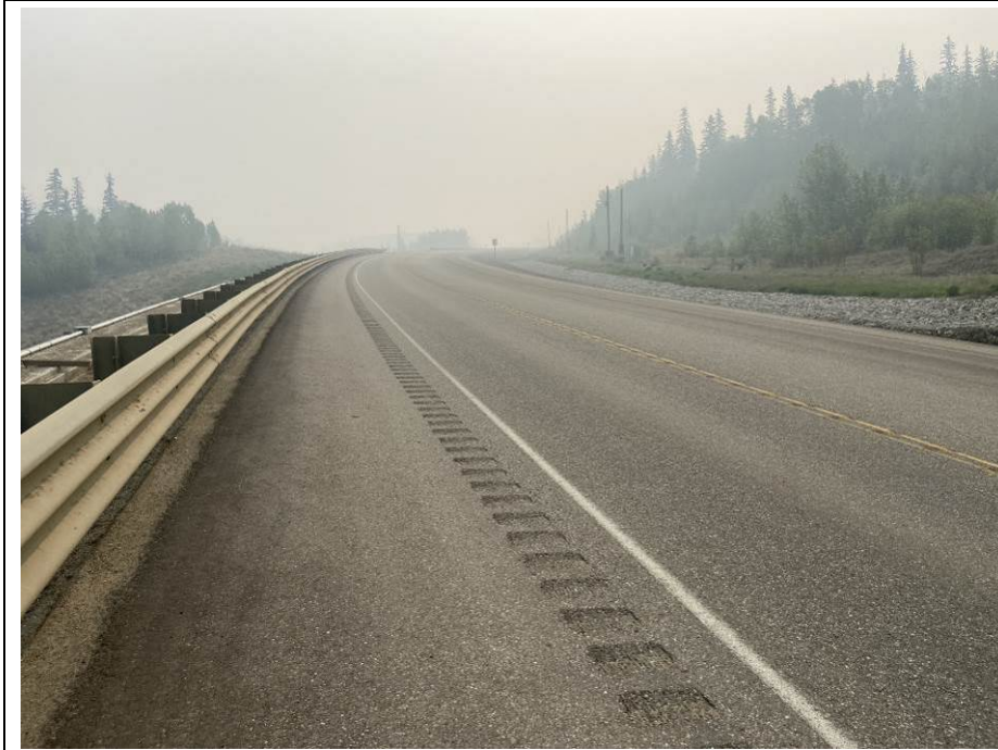
Photo 42-03. Looking east at the replaced highway segment that previously had cracking and settlement across the roadway due to landslide movement (33+210). Road surface was in a good condition at time of inspection and had no observable change from the 2021 condition.
