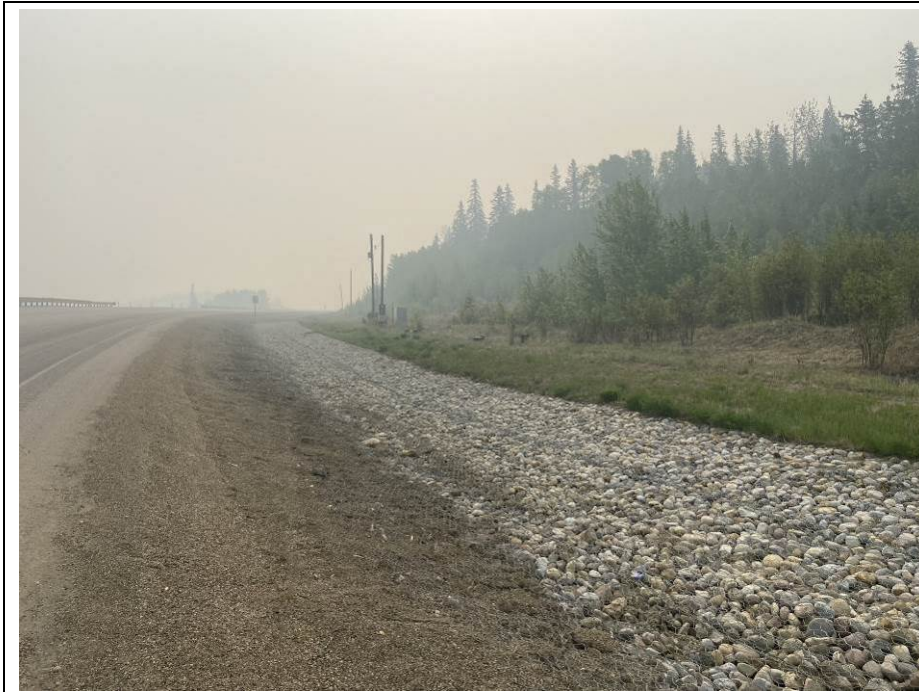
Photo 42-05. View looking east at the gabion mattress installed in the south ditch across the entire site extents to repair previous erosion damage. Minor rill erosion was noted between the road edge and edge of the gabion. No major change within the area east of 33+175 since 2021.
