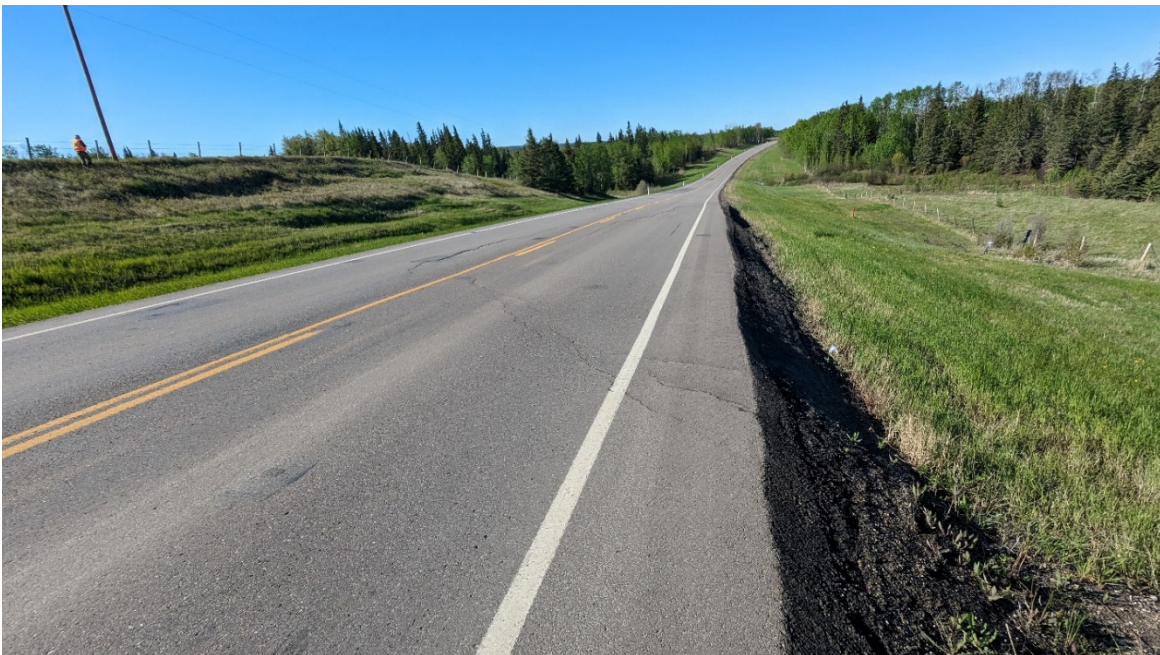
Photo 4 – Looking southeast at a main crack that has resurfaced near the north end of the site.
