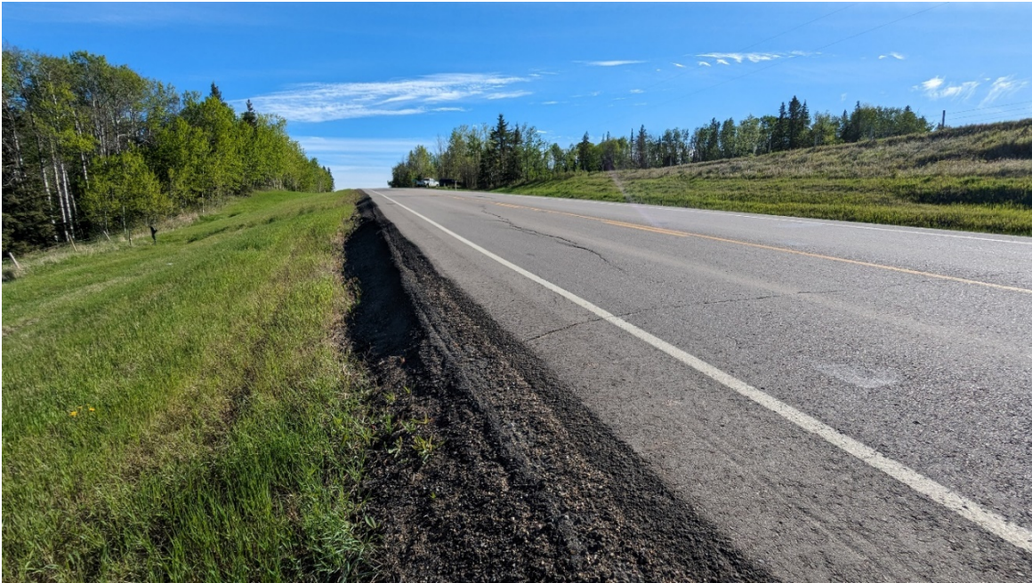
Photo 3 – Looking north at the highway surface at south extent of main crack. Significant thickness of asphalt is visible at the edge of the road.
