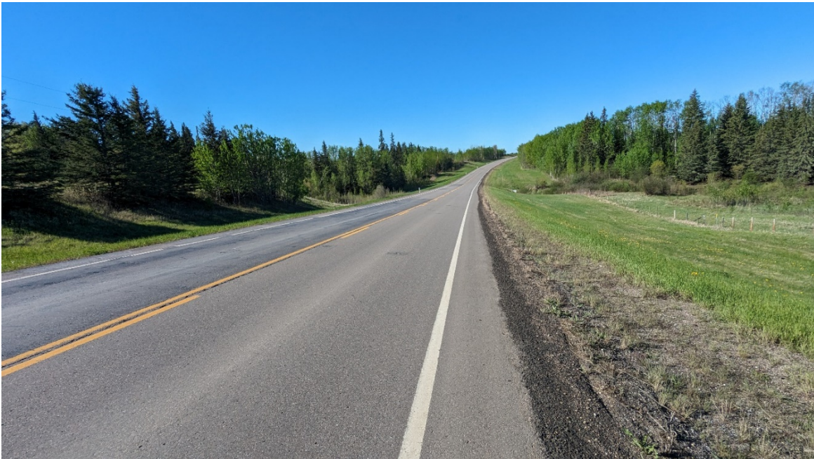
Photo 2 – Looking south at patches along the NBL towards the south end of site.
