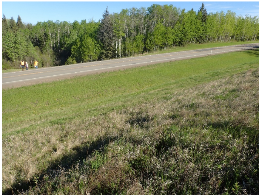
Photo 8 – Looking northwest from the backslope at the observed subsiding area in the pavement.
