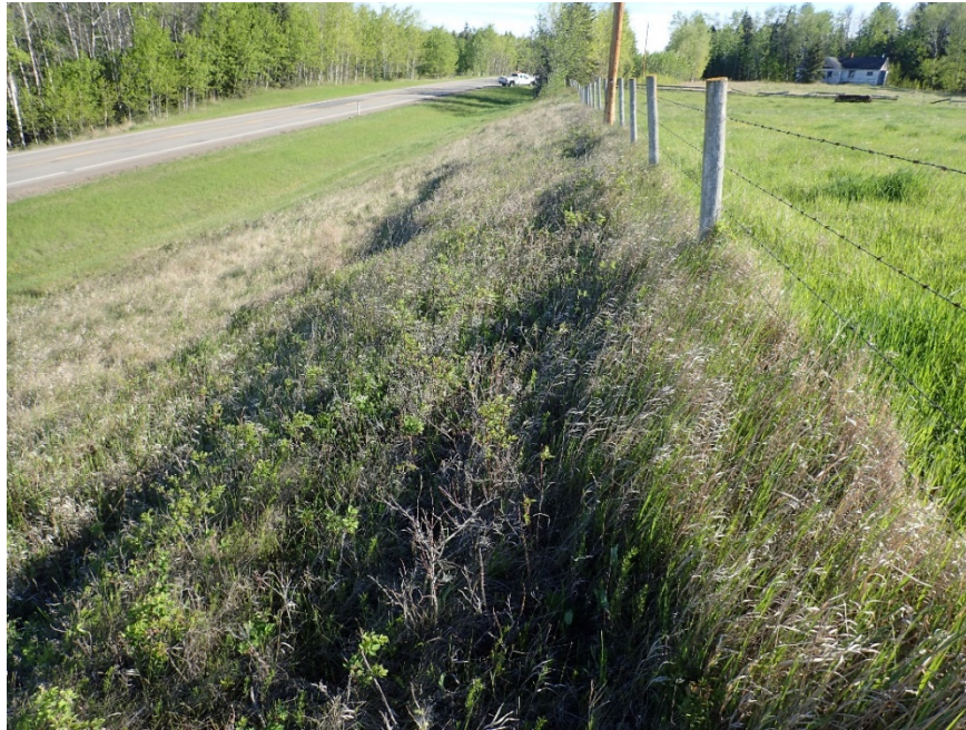
Photo 7 – Looking north at backslope scarp and tension cracks upslope of crack adjacent to fence.
