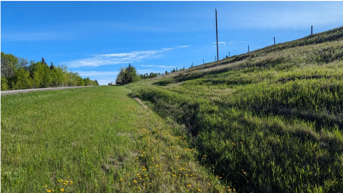
Photo 6 – Looking north at highway east ditch and backslope slumps.
