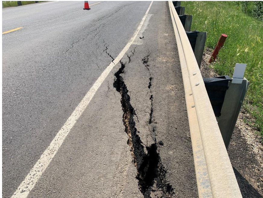
Photo 3. Looking south closer at the crack in the highway shoulder. Photo credit: Nicole Wilder.
