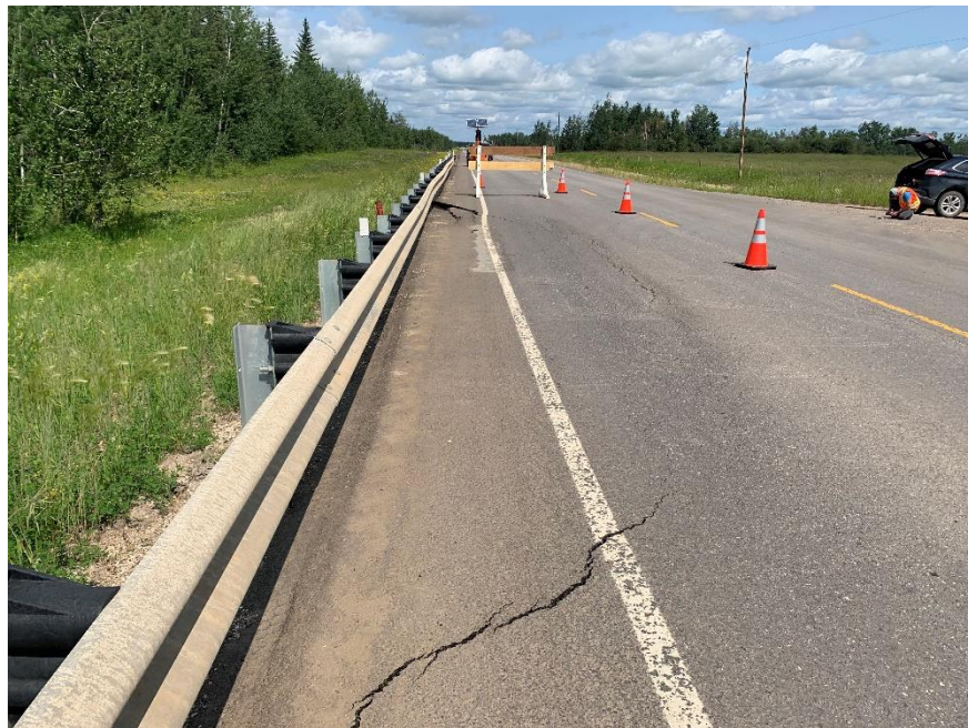
Photo 5. Looking north at the scarp crack arch in the southbound driving lane. Photo Credit: Don Proudfoot.
