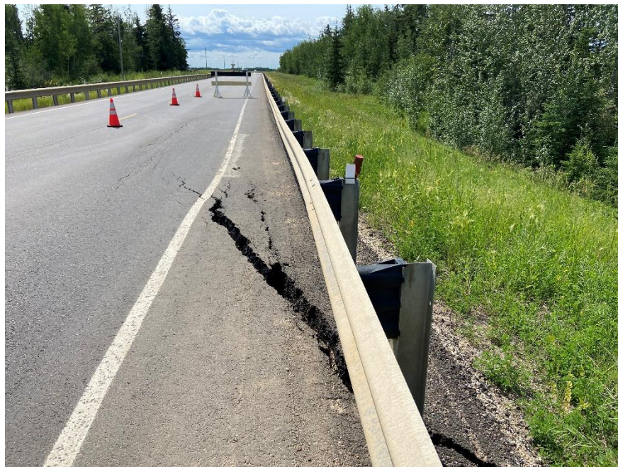
Photo 2. Looking south at crack open to 280 mm wide in the southbound lane shoulder. Photo credit: Don Proudfoot.
