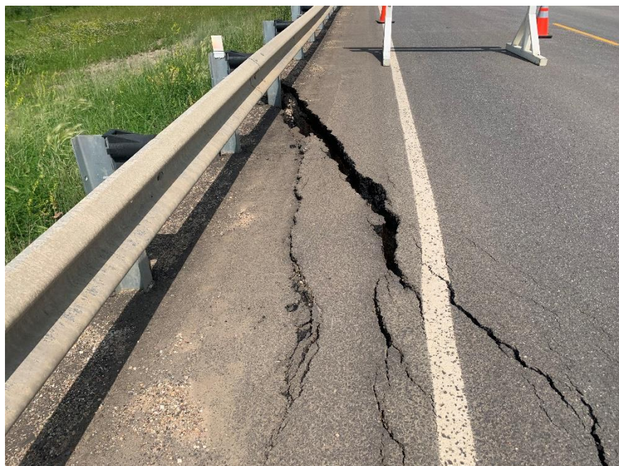
Photo 6. Looking north at the scarp crack leading into the shoulder and embankment. Photo Credit: Nicole Wilder.
