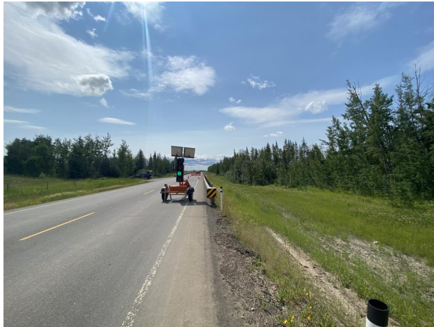
Photo 1. Looking south at traffic lights set up for the one lane closure. Photo credit: Don Proudfoot.
