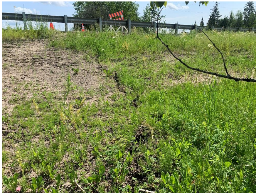
Photo 4. Looking east at the scarp crack that continues in the highway embankment. Photo credit: Nicole Wilder.
