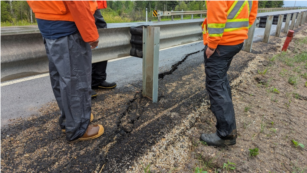
Photo 5: A close look at open cracks on the highway SBL shoulder.
