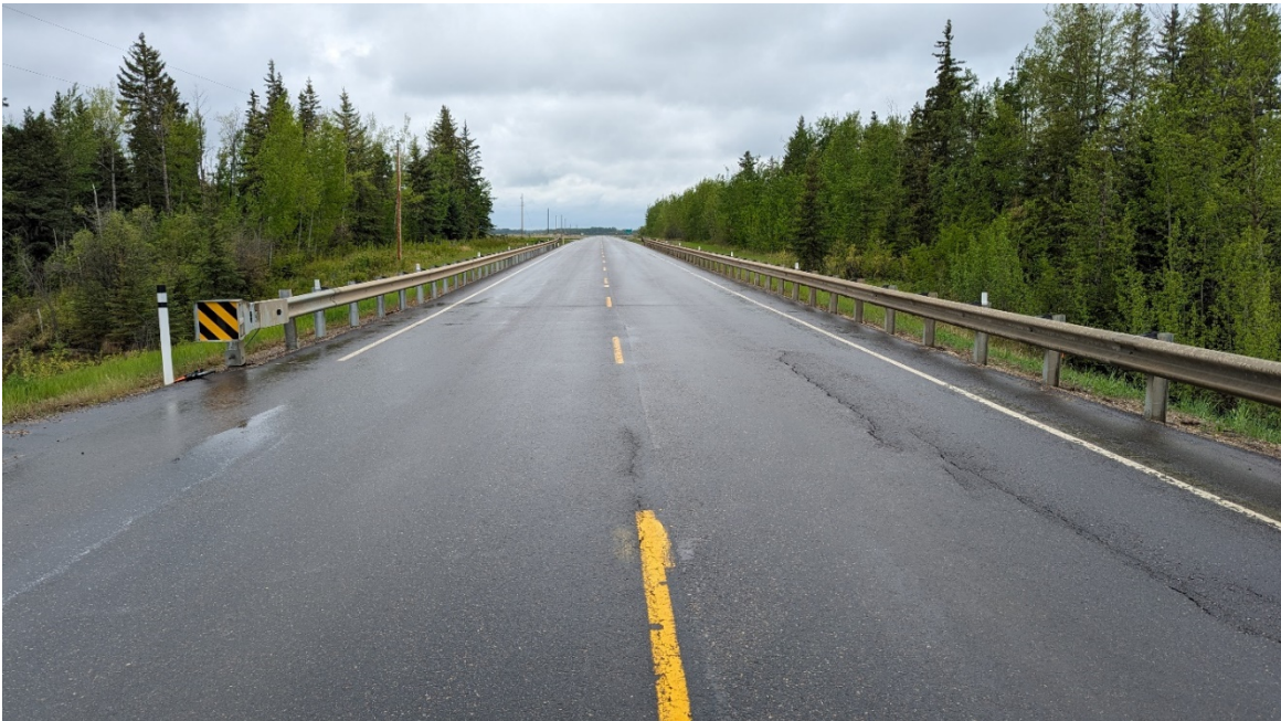
Photo 2 – Looking north along the centerline of highway. Tension cracks resurfacing on southbound lane. New guardrails installed on both sides of the highway.
