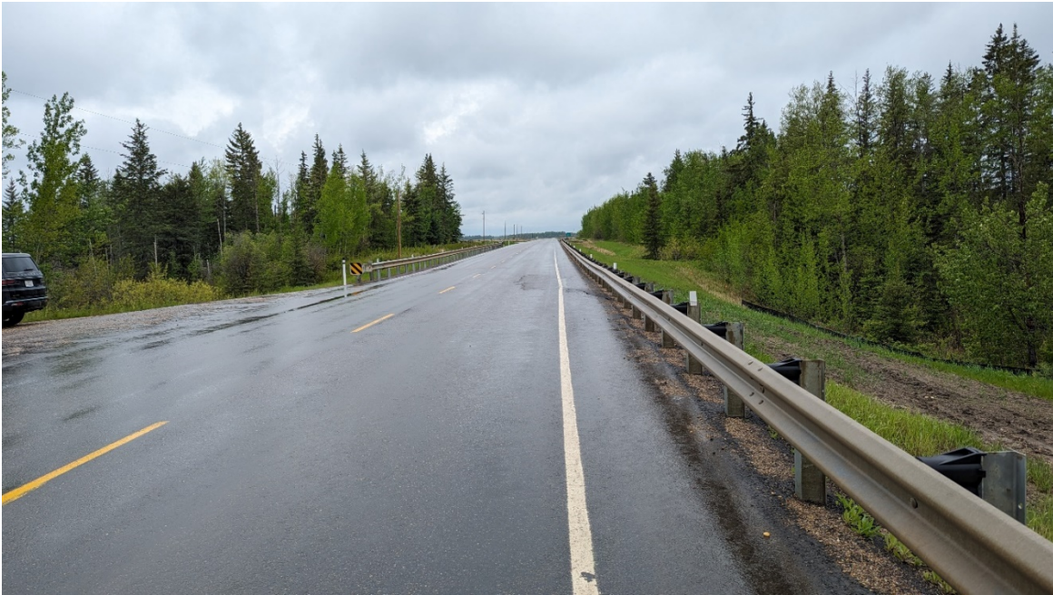
Photo 1 – Looking south along southbound lane from the north end of site. The scarp that has retrogressed into the highway is visible on the shoulder.
