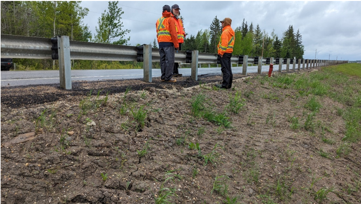
Photo 6: Looking southeast at crack that has retrogressed towards the highway.
