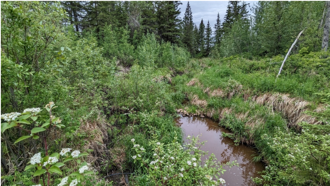
Photo 8: Looking west from above the culvert outlet location at creek and bank erosion.
