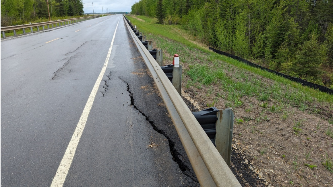
Photo 3: Looking south at scarp crack that retrogressed into the highway. Tension cracks observed along the southbound lane.
