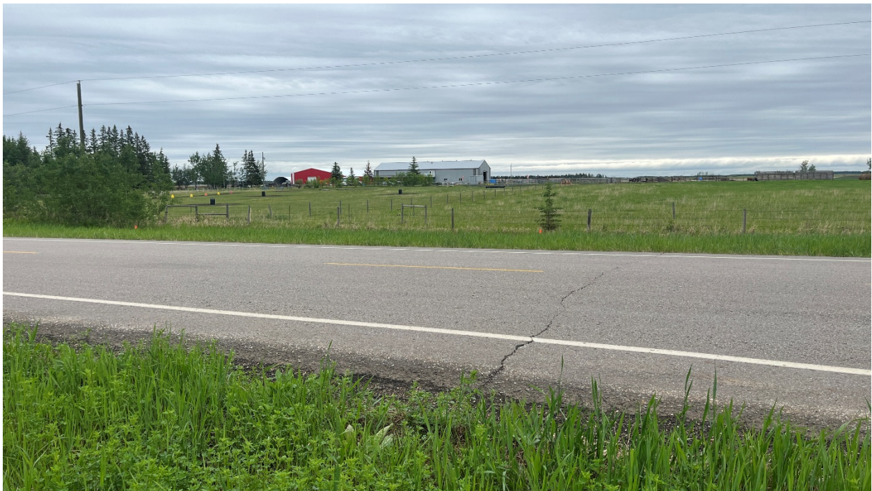
Photo 4: Looking northeast at transverse cracking on the pavement at the middle portion of the site.
