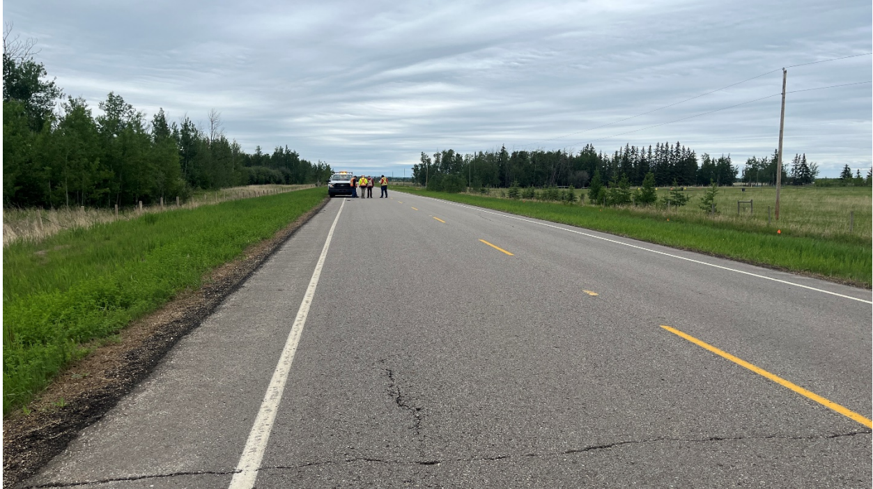
Photo 3: Looking north from the south end of the site near the 1800 mm diameter culvert.
