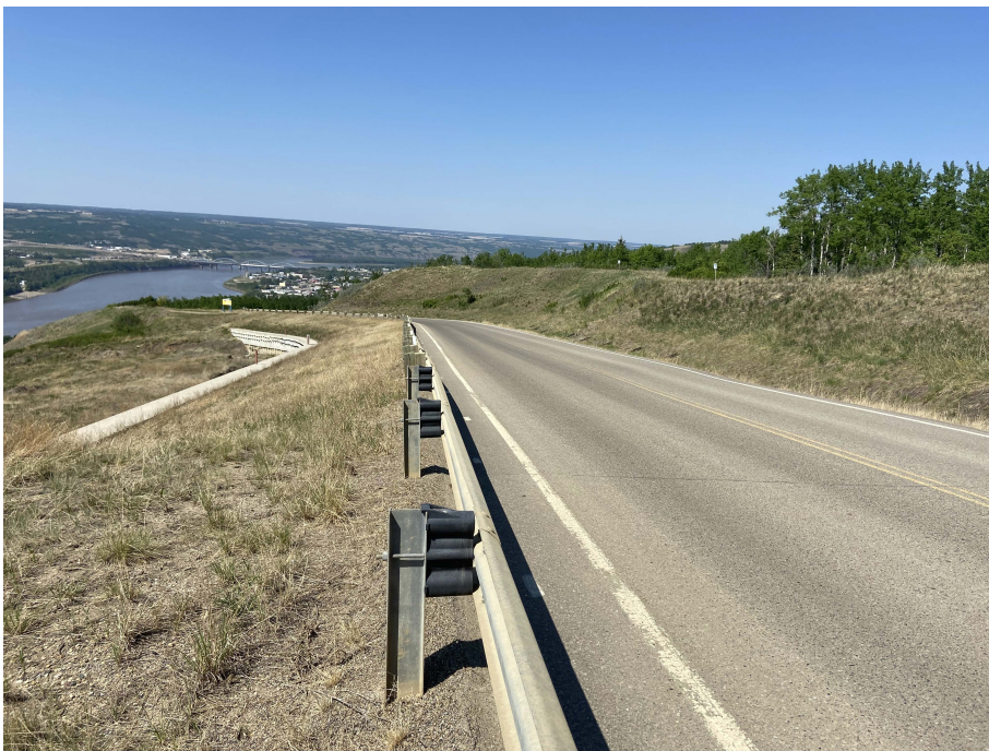
Photo 3. Looking northwest from south end of the Sunshine pile wall at km 58.200 along the highway. No damage to the ACP surface was observed.
