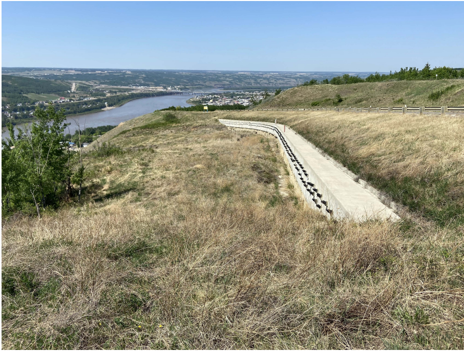
Photo 2. Looking northwest from south end of the Sunshine pile wall at km 58.200. No major visible changes from the 2021 condition.
