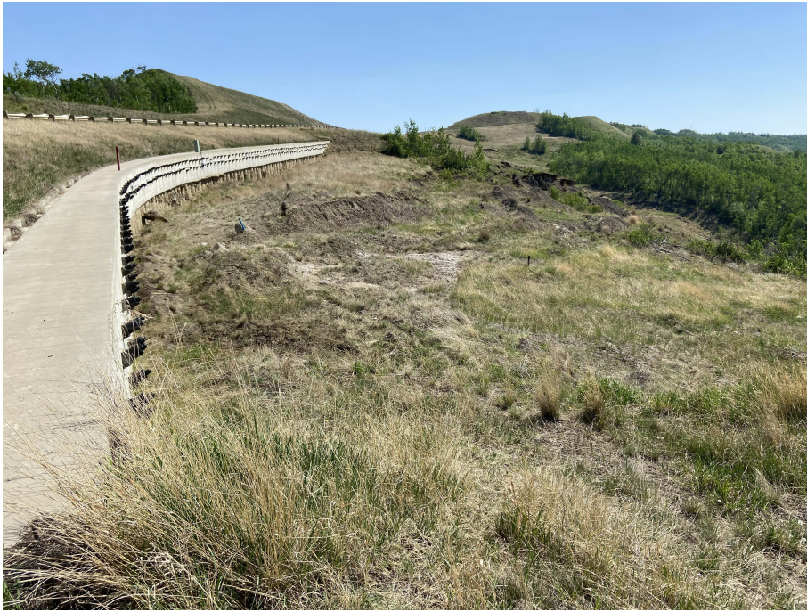
Photo 4. Looking southeast along the pile wall at km 58.33. Head scarp cracks immediately below the wall appear unchanged since the 2021 inspection.
