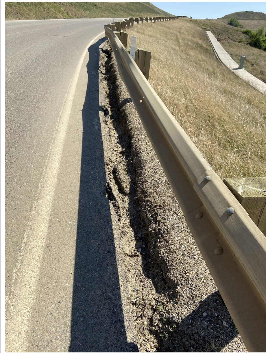
Photo 1. Looking south along the SBL of Hwy 744:04 at km 58.35 at the north end of the Sunshine pile wall. An erosion gully has developed parallel to the edge of the ACP.
