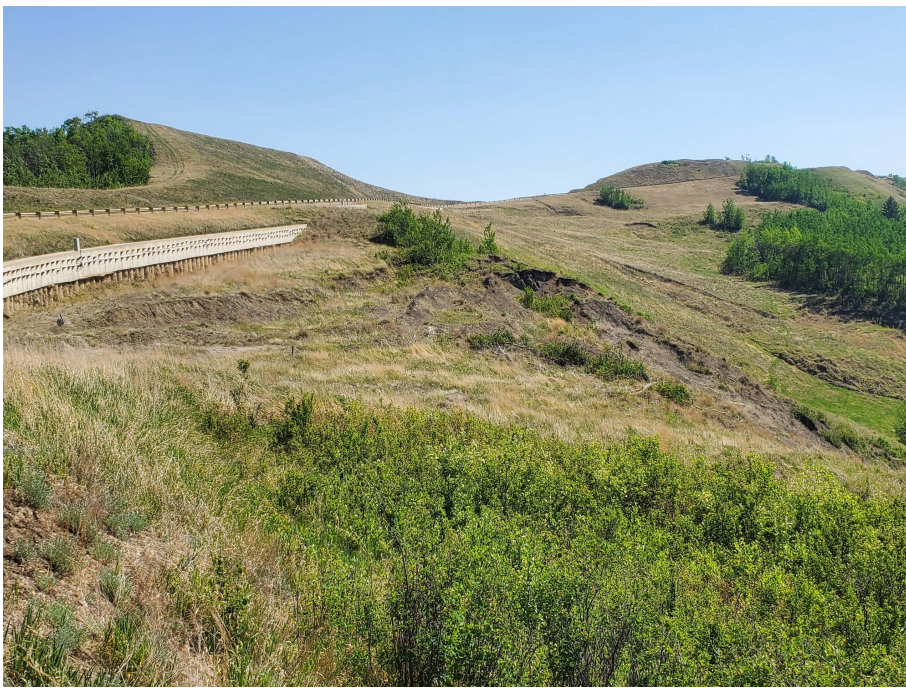
Photo 5. Looking southeast at the lower slide area below the wall. Active ongoing slide movement within the lower slope.
