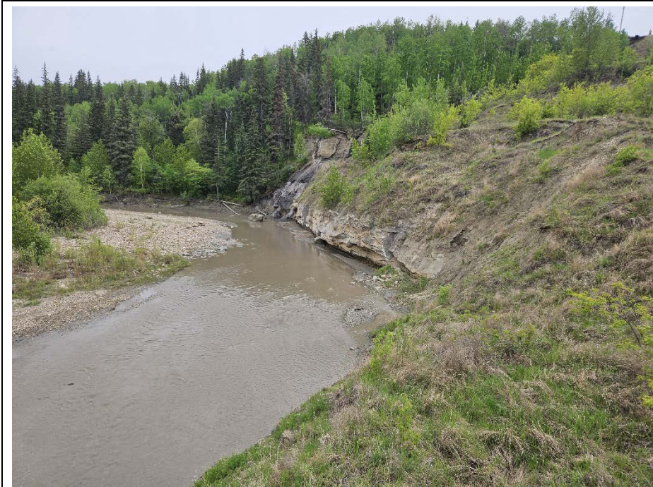
Photo 10. Looking south towards the base of the lower slide and bedrock exposure at the river. Some minor lower slide activity and active erosion of slide materials entering over the bank. No major change from the 2023 condition.
