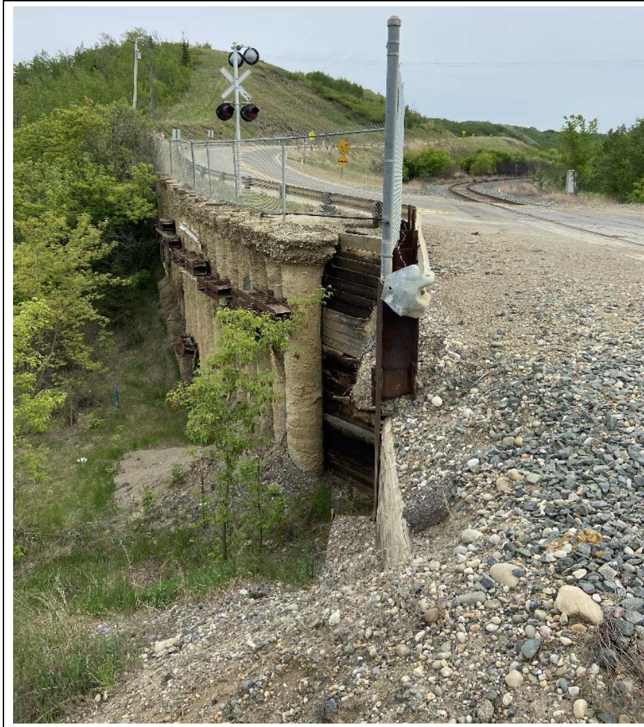
Photo 1. Looking southeast from the north end of the CNR pile wall. Grout / lean concrete overflow from the 2022 repair of the void behind the wall is visible at the toe of the wall.
