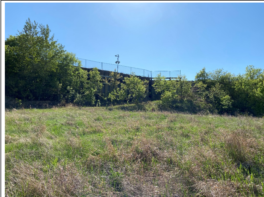
Photo 11. View towards the lower slope area downslope from the base of the pile wall and immediately upslope of the main slide scarp monitored by S110-17. No visible indications of landslide movement were observed in this area and conditions were similar to 2023 inspection.
