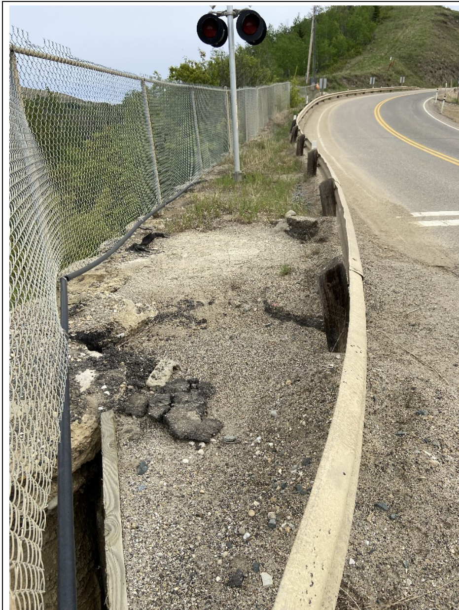
Photo 2. View of the repaired area behind the pile wall where erosion voids formed in 2020 and 2022. The repair involved geotextile supported by wood cribbing and backfilled with grout/lean concrete. The voids were a result of soil loss between the piles, and over 5 m in depth prior to repair. The repairs appeared to be working as intended during the 2024 inspection and no visible signs of void formation were identified along the ground surface behind the wall.
