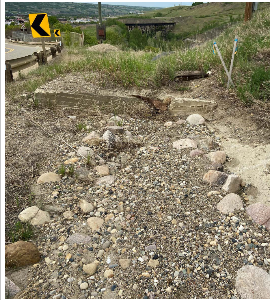
Photo 12. Buildup of eroded ditch sediment (sand and gravel) at the down pipe trunk inlet.
