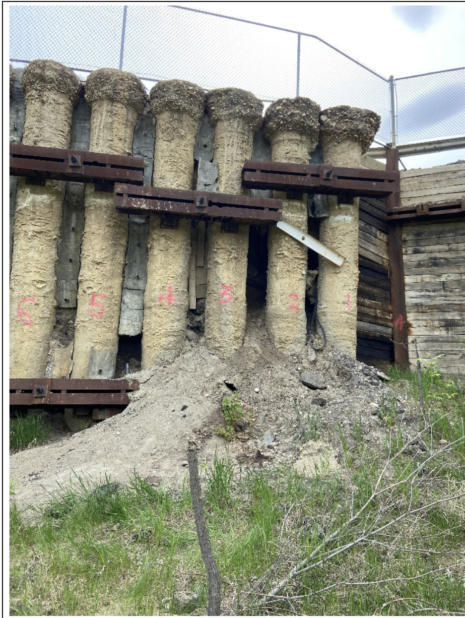
Photo 3. Looking south at the soil loss between the northernmost piles (1 to 5) of the CNR pile wall north of Hwy 744:04 at km 59.61. Increased buildup of soil spalling between the piles since 2023. Note wood cribbing set behind the piles to help contain the grout backfill for the void repair; however, some grout still did flow through and has set along the toe of the piles.
