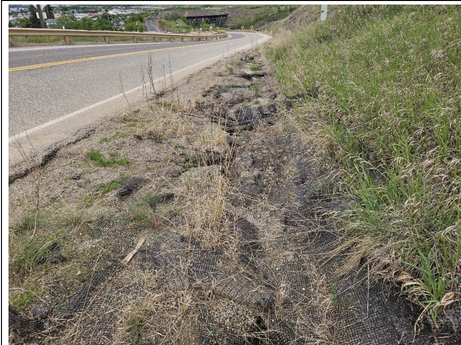
Photo 8. Looking north towards the east ditch with previous erosion damage that was repaired in 2022 (regraded, with TRM and ditch barriers). Vegetation was not well established and there was a minor erosion channel starting to develop within the ditch bottom and some barriers were partially undermined.
