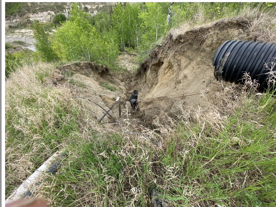
Photo 4. Looking northeast at break in CNR CPP Trunk pipe and erosion gully at crest of the Heart River valley slope. More pipe segments have fallen into the gully since the 2023 inspection.
