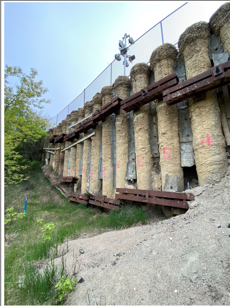
Photo 13. Looking towards the southeast at the base of the pile wall with spalling concrete between the piles.
