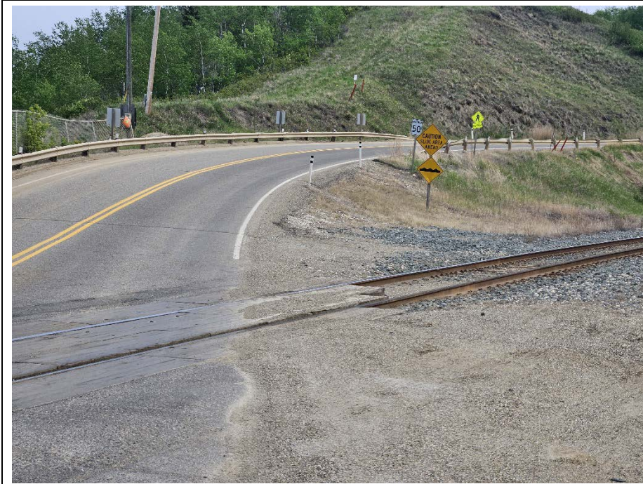
Photo 7. Looking east at previous embankment area with erosion gullies and rill erosion that was repaired in 2022. Sideslope repairs appeared effective and similar to the 2023 conditions.
