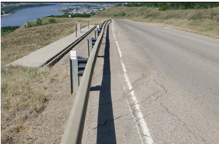
Photo 8. Looking northwest at the highway above the "Makeout" pile wall. Some increased dip around the SBL shoulder near the middle and south end of the wall and ACP cracking was slightly worse relative to the 2021 condition.
