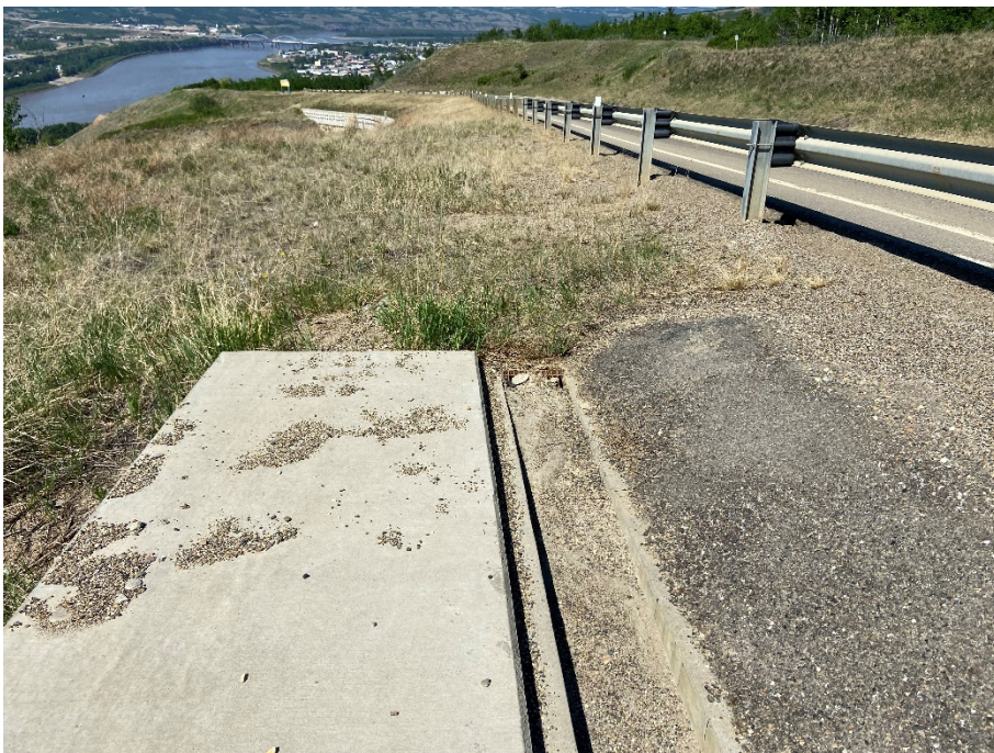
Photo 10. Looking at the north end of the top of the “Makeout” pile wall. Drainage trough inlet was relatively clear and functioning.
