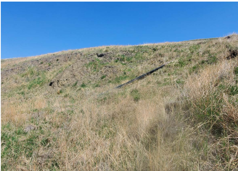
Photo 6. Looking at the north flank of the lower slide area between the pile walls. Seepage from a disconnected drainage pipe is causing erosion and exacerbating slide movement. No major changes from the 2021 condition.
