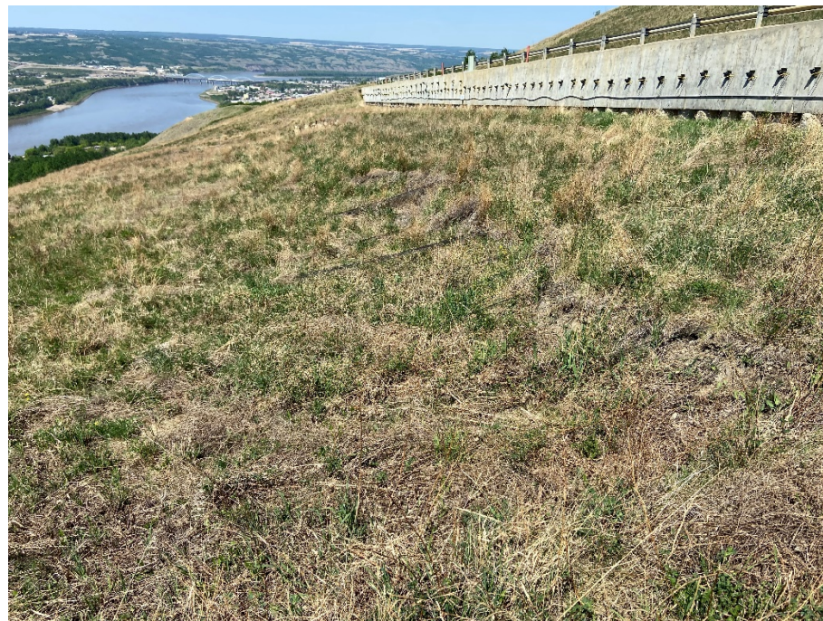
Photo 4. Looking northeast from below the north end of the km 58 pile wall. The old landslide scarps below the pile wall that were regraded in 2015 have ongoing movement. There was a tension crack along the downslope edge of the old pile wall with up to 0.3 m of drop.
