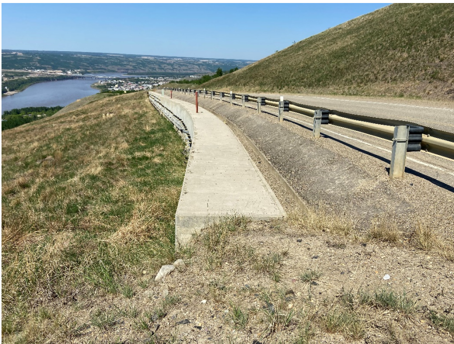
Photo 2. Looking northwest from the south end of the km 58 pile wall. The ACP shoulder protective cover was in good condition. No significant changes were noted downslope of the wall at this site relative to the 2021 condition.
