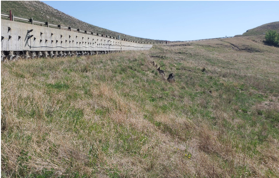
Photo 5. Looking south at the landslide scarps downslope from the km 58 pile wall (km 58.07). A new tension crack was observed in this area with up to 0.4 m drop. The old piles are exposed up to 2.0 m in height.
