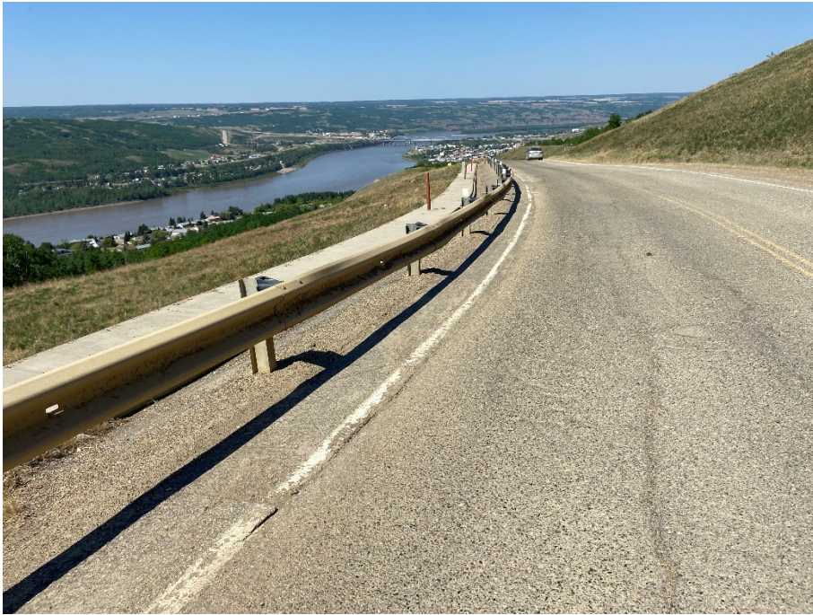
Photo 1. Looking northwest from the SBL shoulder of Hwy 744:04 at km 57.96 along the guardrail above the km 58 pile wall. There have been no major changes in the cracks in the ACP within the southern half of the wall since 2021.
