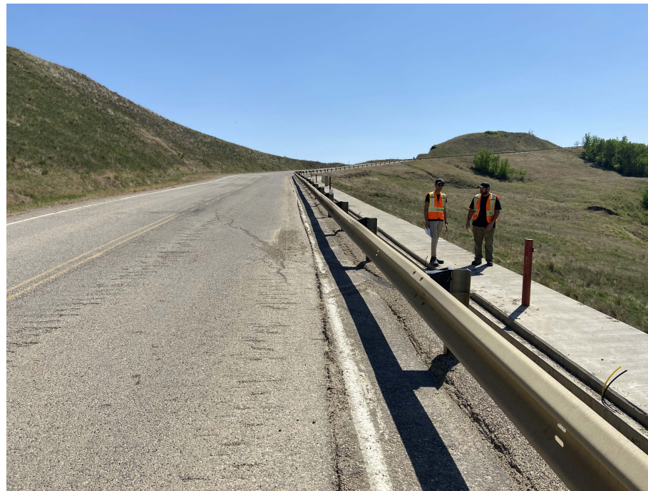
Photo 3. Looking south from the north end of the km 58 pile wall. Slightly worse crack and dip within the ACP directly behind the wall but overall road condition has not significantly changed since the 2021 condition.
