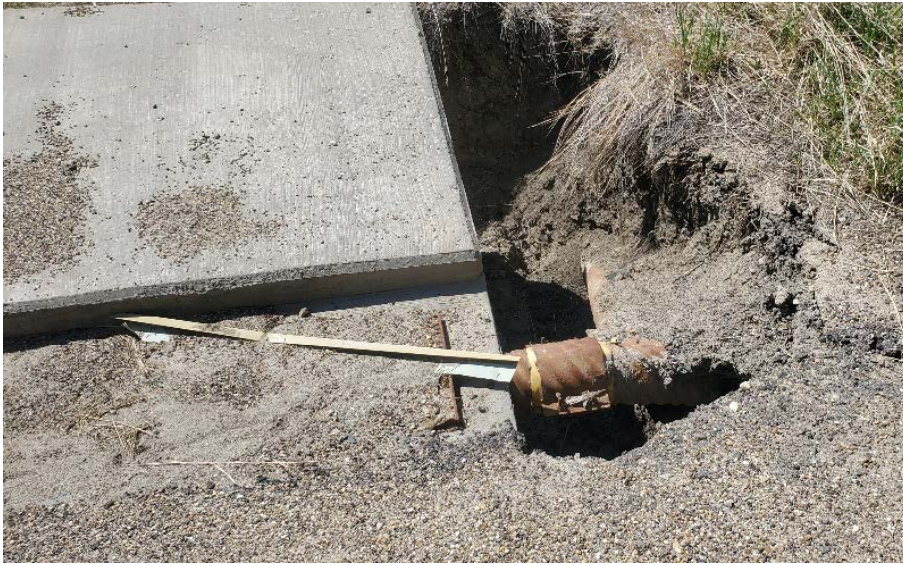
Photo 7. Looking at the north end of the km 58 pile wall where the drain outlet has become blocked and caused water overflow and scour exposing the subdrain and gutter pipes.
