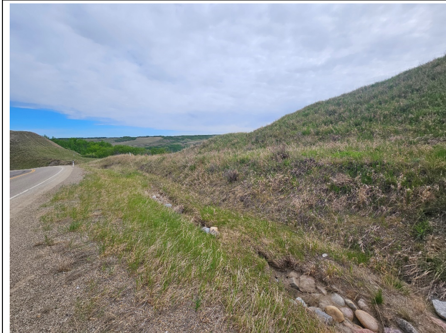
Photo 2. Looking northeast along the east ditch near km 57.65 where there is ongoing ditch erosion that has become slightly worse since 2023.
