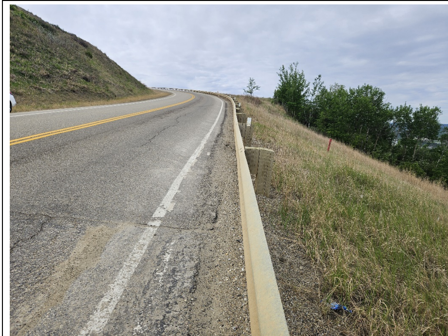
Photo 1. Looking southwest along the centerline of Hwy 744:04 at km 57.65 near the north end of the 2014-2015 realignment. Cracks have not significantly expanded but localized settlement (estimated up to 150 mm) is more apparent at the shoulder relative to the 2023 condition.
