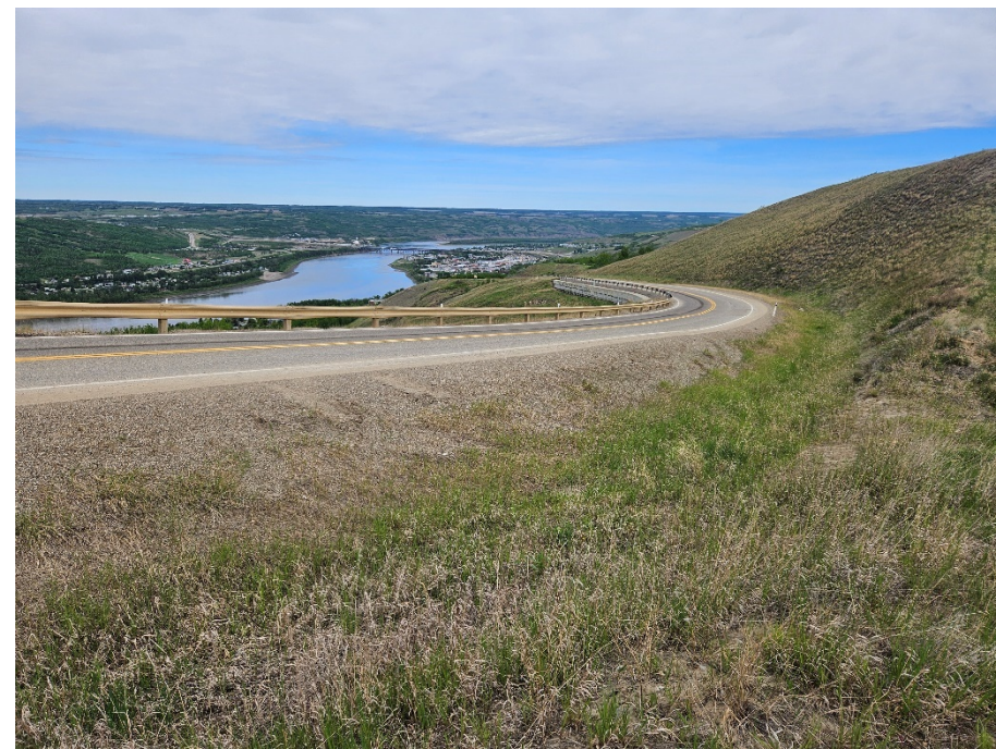
Photo 6. Looking north along the east side of Hwy 744:04 at km 57.8 and upslope of the landslide movement towards the Heart River. No new cracks were apparent in the pavement or ditch area upslope from the backscarp.
