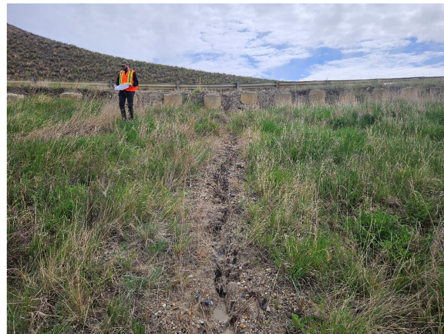
Photo 5. Looking north along the west side of Hwy 744:04 at protruding piles near km 57.9. Max drop of 1.8 m below top of pile (unchanged since 2023). An erosion rill has formed from runoff between the piles.
