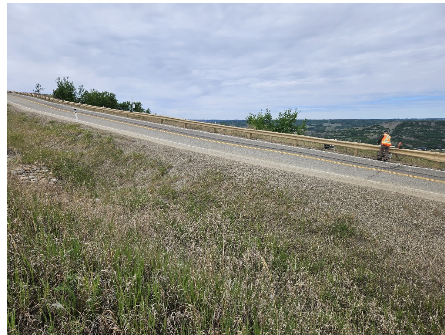
Photo 7. Looking southwest along Hwy 744:04 from km 57.85 at the crack and dip across the road. No significant visible change from the conditions observed in 2023.
