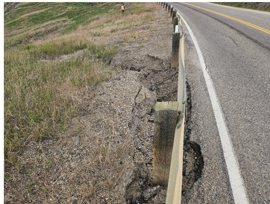
Photo 3. Looking north at gully erosion on the west side of the highway near km 57.75. The gully is up to 1.2 m wide and 0.8 m deep and is slightly worse from the 2023 condition.
