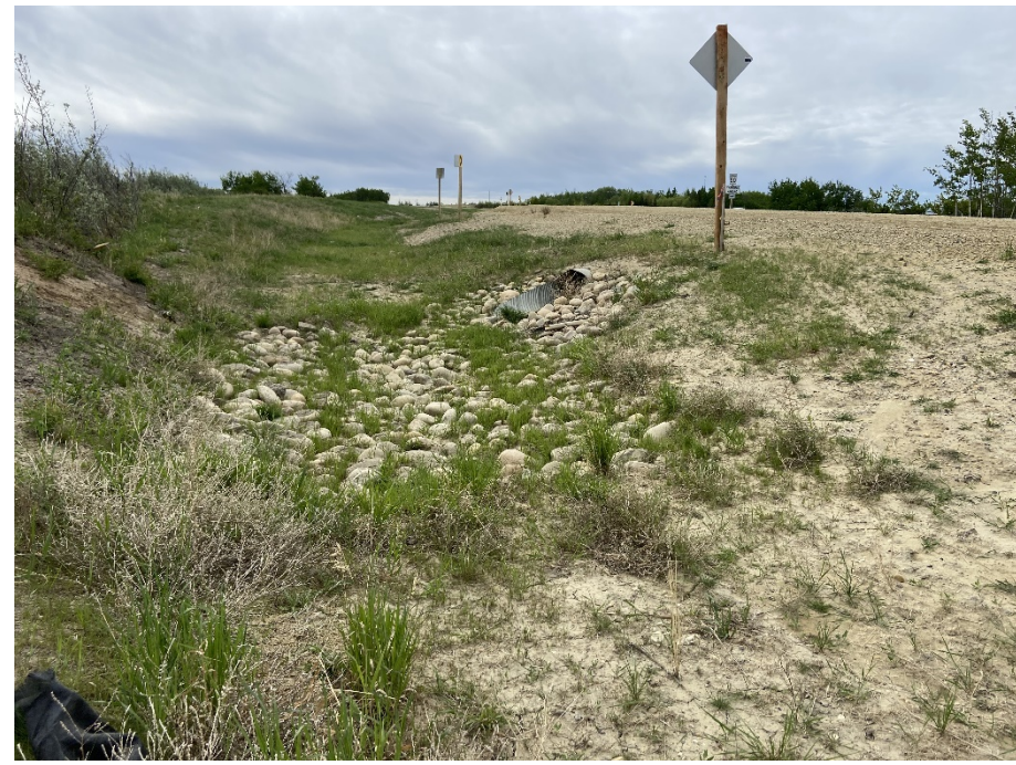
Photo 30-09. Looking south along the east ditch of the new gravel realignment and new culvert outlet (km 57.52). There is a low spot within the ditch that should be fixed by regrading for an approximately 20 m section north of the outlet to prevent ponding. No ponding was observed in 2024.
