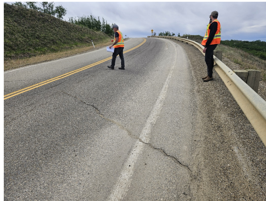
Photo 30-07. Looking south along SBL of Hwy 744:04 at km 57.68. Arc-shaped cracking more prominent in SBL within the downslope extents of Slide 1A. Dip was more pronounced relative to the 2023 condition and cracks have started to extend into NBL.
