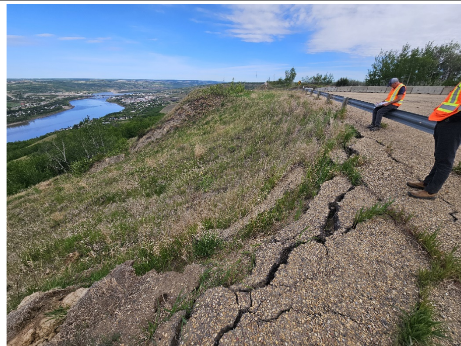
Photo 30-02. Looking north along backscarp of Slide 2A (previously Slides 2 and 3) which has a minimum offset of 0.45 m from the parking lot guardrail. Some localized main scarp retrogression at south end, flank erosion and additional pavement cracking since 2023. Tension cracks are now at the guardrail.
