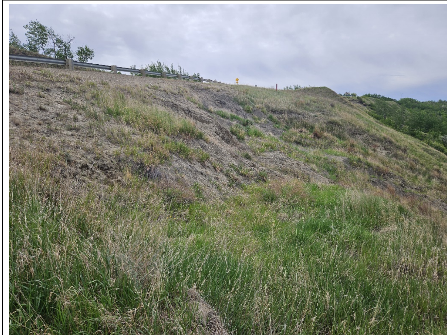
Photo 30-06. Looking south at Slide1A (near KM 57.65). Ongoing downslope movement and erosion at the main scarp and south flank; however, no major change from the 2023 condition.
