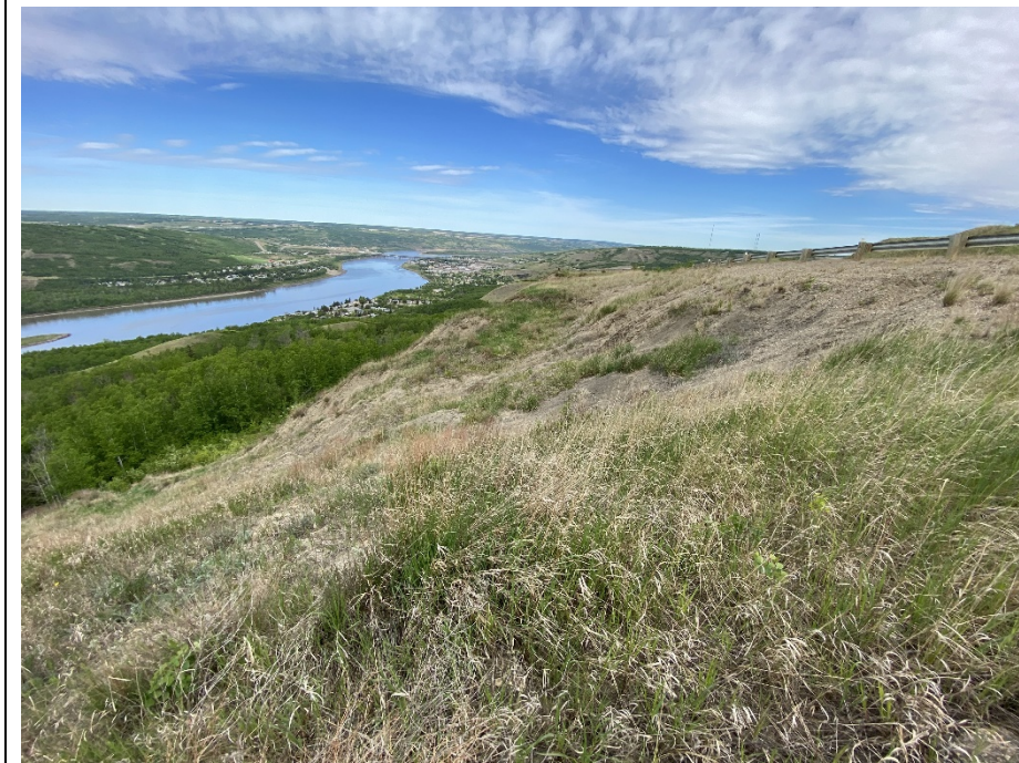
Photo 30-05. Looking north from downslope of the SBL of Hwy 744:04 near km 57.63. Increased down drop within the disturbed slide mass of Slide 1A. Main scarp had minor retrogression since 2023 and is offset a minimum of 2.0 m from the guardrail (unchanged from 2023).
