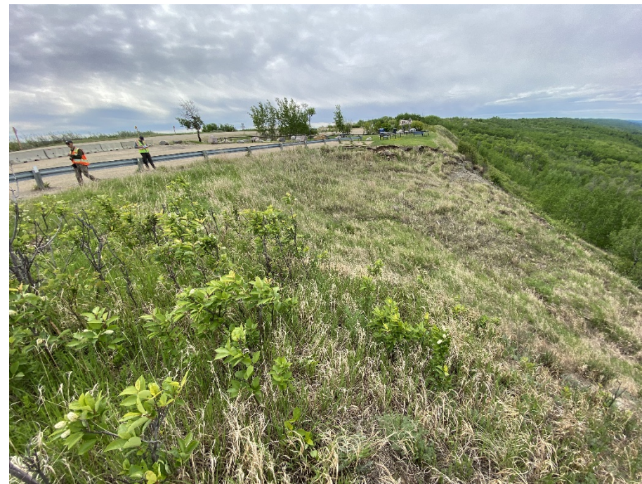
Photo 30-03. Looking south towards the upper part of Slide 2A. South flank had most activity since 2023 within increased erosion and minor retrogression. Ongoing movements occurring further downslope, primarily involving shallow earth flows.
