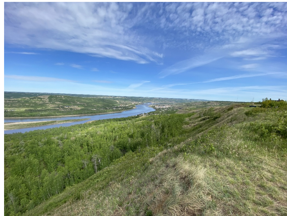
Photo 30-01. Looking north towards the Slide 4 area from the south end of the site. No change to the slide in this area has been observed over the last several years and it is well vegetated.
