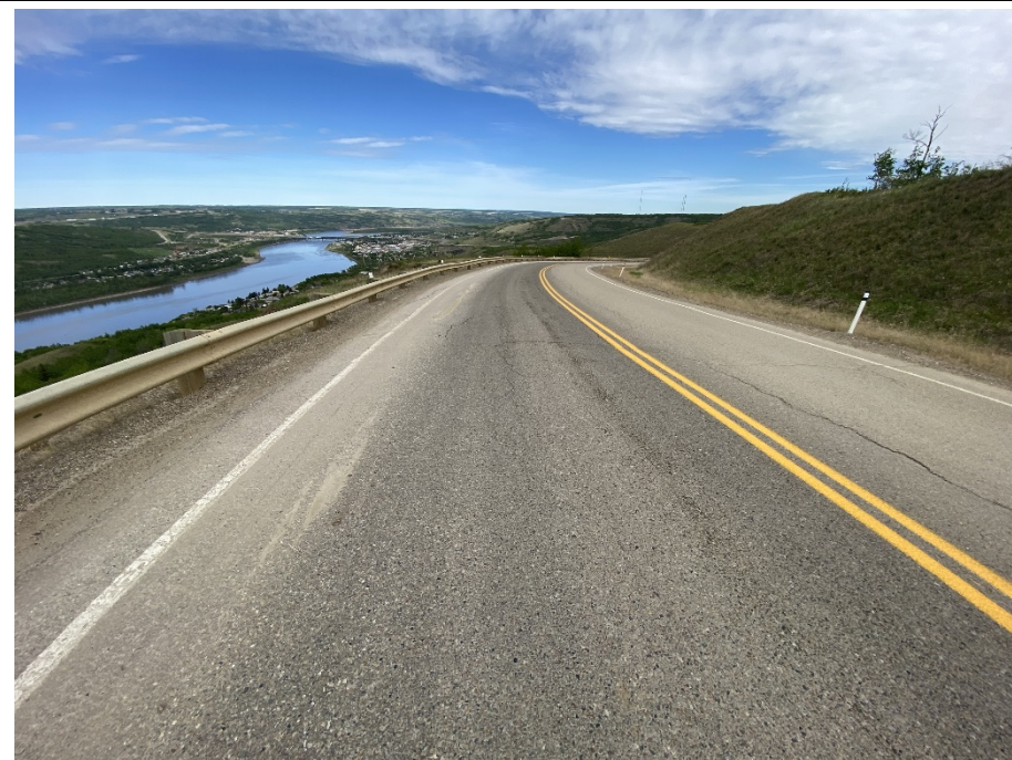
Photo 30-04. Looking north along the SBL of Hwy 744:04 near km 57.65 at south end of 2015 realignment. Transverse cracks have formed joining the previous longitudinal crack in the NBL to form arc-shaped crack within the downslope extents of Slide 1A. Cracks have extended into the NBL.
