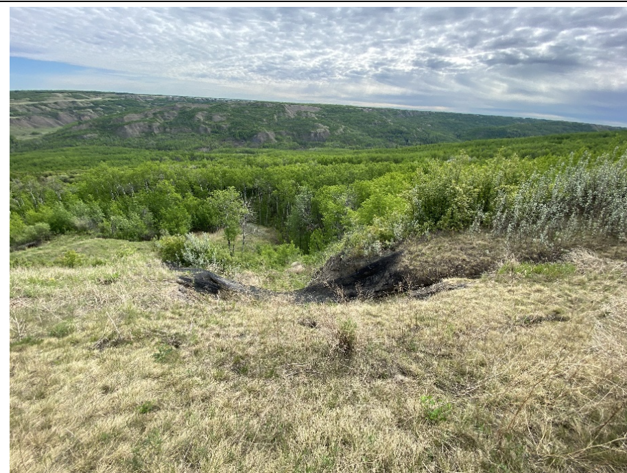
Photo12- 10. Active gully erosion within the top of Main Slide 4. Erosion damage at the gully headwall appeared worse relative to the 2023 condition and a new tension crack had developed 2 m upslope from the gully headwall.
