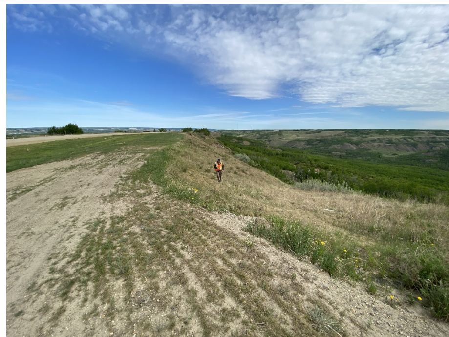
Photo 12-08. Looking north from south end of the former Slide 4 repair area. Overall repairs from 2014 are performing well. Overall slope is well vegetated and with no visible indications of new slide development within the granular backfill slope. Old highway alignment has grass development.
