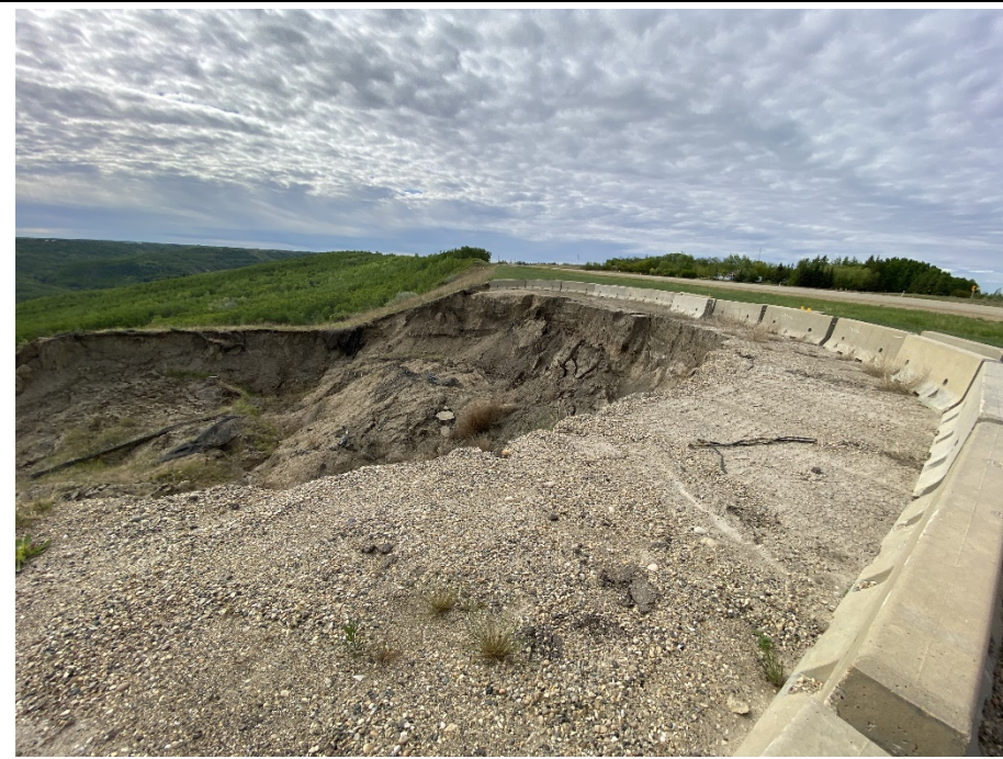
Photo 12-01. Looking south from north side of Main Slide 1A. There is ongoing retrogression and erosion primarily within the southern half of the main scarp and south flank. Tension cracks were observed 0.8 m behind the main scarp. Main scarp offset from the edge if the gravel realignment is approximately 35 m (unchanged from 2023).
