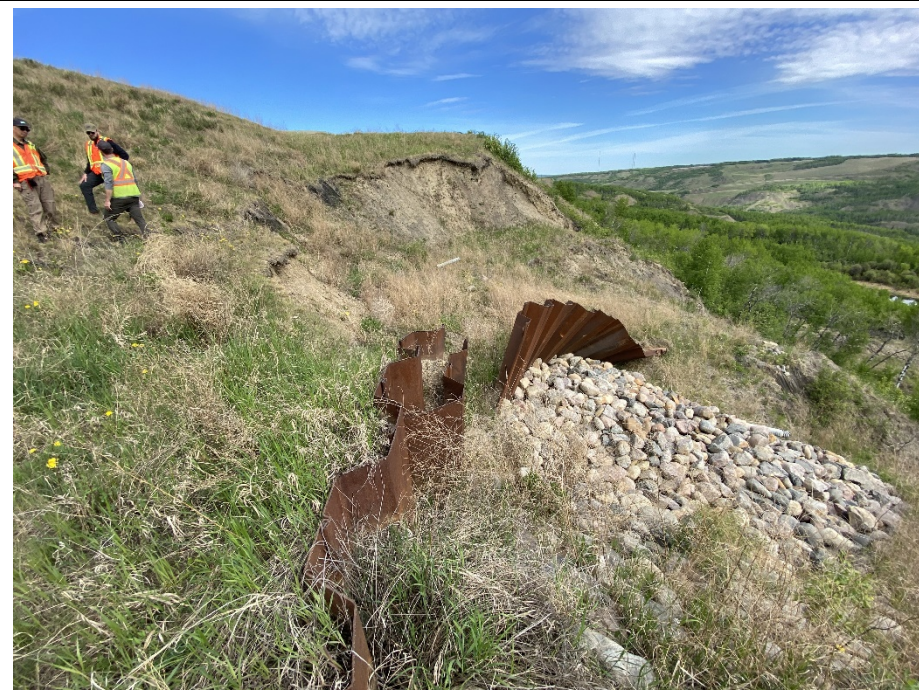
Photo 12-06. Looking north at the former Slide 2 area with ongoing downslope slide movement and erosion of the upper scarp. No major changes observed since 2023. Deflection of the sheet piles appears similar to the 2023 condition.
