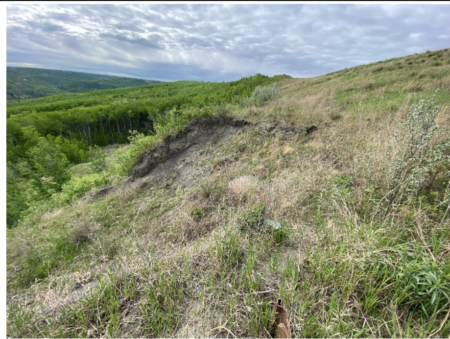
Photo 12-05. Looking south at Main Slide 2.1 south of the sheet pile wall. No major retrogression of the scarp at this location since 2023.
