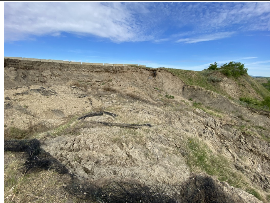
Photo 12-03. Looking upslope towards the west at the main scarp and slide runout area of Main Slide 1A from the lower south flank.
