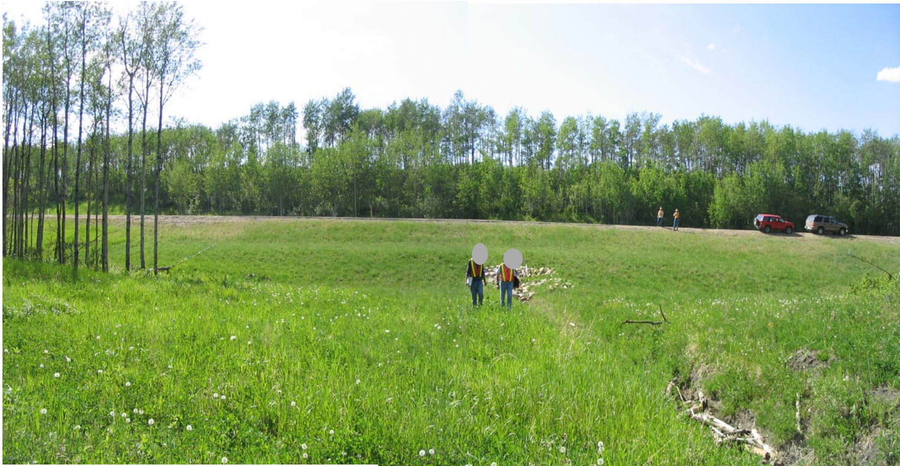
PHOTO #2 : LOOKING NORTHWEST AT CULVERT OUTLET. NOTE : GOOD VEGETATION GROWTH SINCE LAST YEAR OVER REPAIRED AREA.
